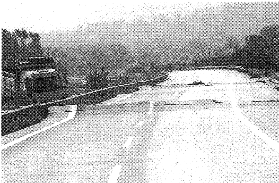
Figure 30: Damage to E80 motorway carriageway caused by fault trace.
