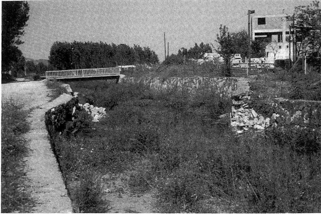
Figure 8: Right-lateral offset (ca 1.5 m) of a canal near Izmit. This photo shows just one or two fault traces at this locality; the total lateral displacement exceeding 2.5 m.
