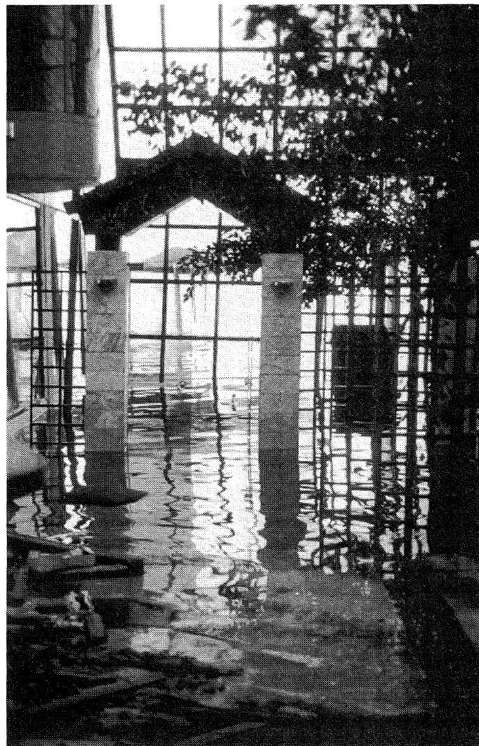
Figure 14: Flooded atrium of hotel at Lake Sapanca caused by soil liquefaction and lateral spreading. The building has settled and moved out into the Lake.
