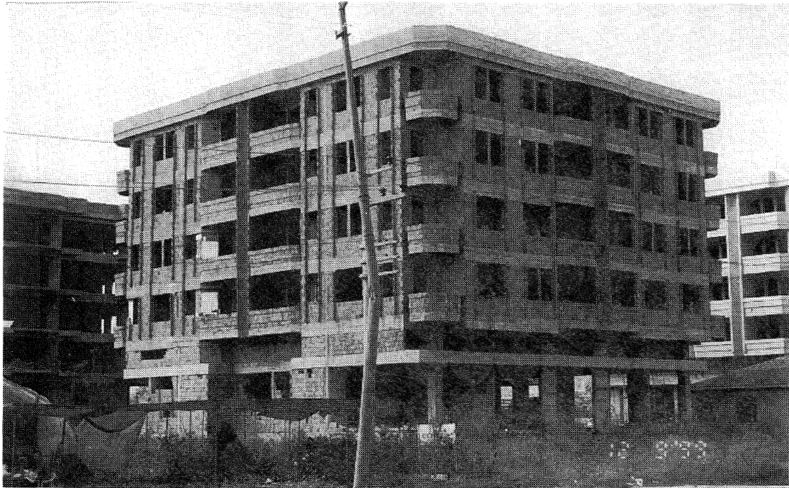
Figure 19: Typical apartment building under construction showing setback concrete columns, hollow brick infill in progress and soft storey ground floor.
