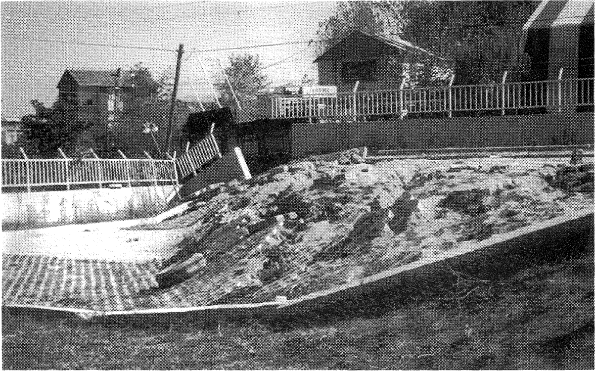
Figure 6: In the Golcuk area, a right-step, or releasing bend, in the fault trace resulted in tectonic subsidence, instead of lateral displacement, across the fault. The tectonic down-drop is expressed in this photo as a normal fault scarp (1-2 m high) in cobblestone pavement.
