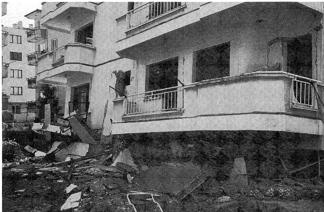
Figure 20: Near new apartment building with collapsed ground floor.
