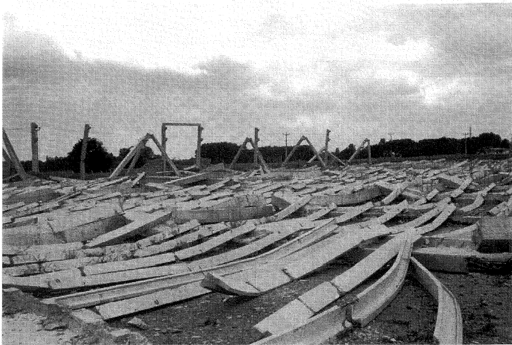
Figure 28: Collapsed precast concrete building near TEM Adapazzari exit.
