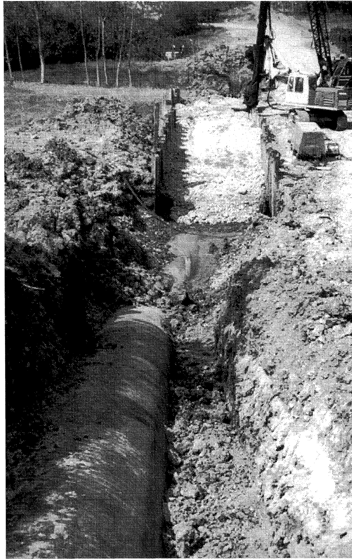
Figure 17: Main water pipeline supplying Izmit after repair. Note the right lateral offset where the pipe crosses the fault trace.
