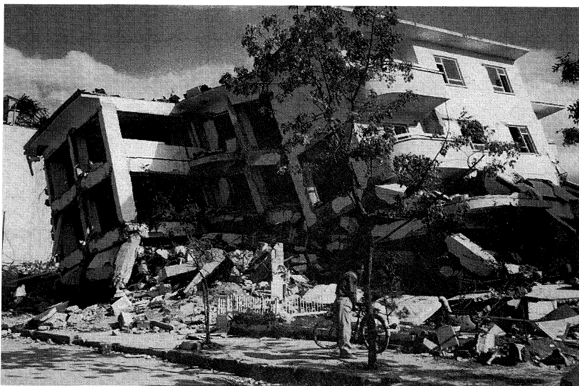
Figure 18: Typical collapsed masonry infill, reinforced concrete frame apartment block.
