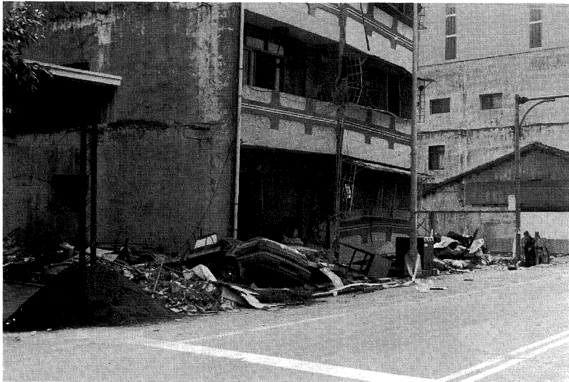
Figure 5.7: Weak storey collapse, Chi-Chi.
