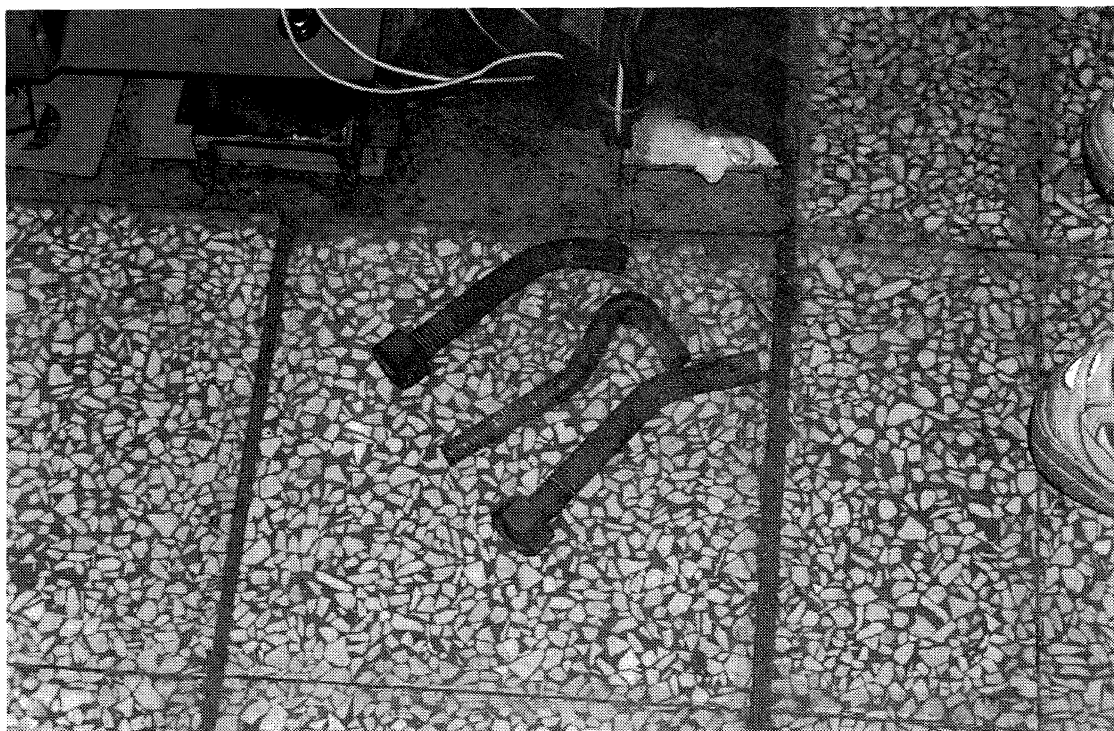
Figure 5.22: Detail of failed holding down bolts that allowed cabinets to topple.
