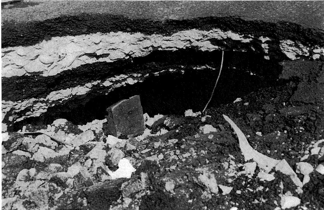
Figure 3.18: A typical liquefaction feature behind a bridge abutment.
