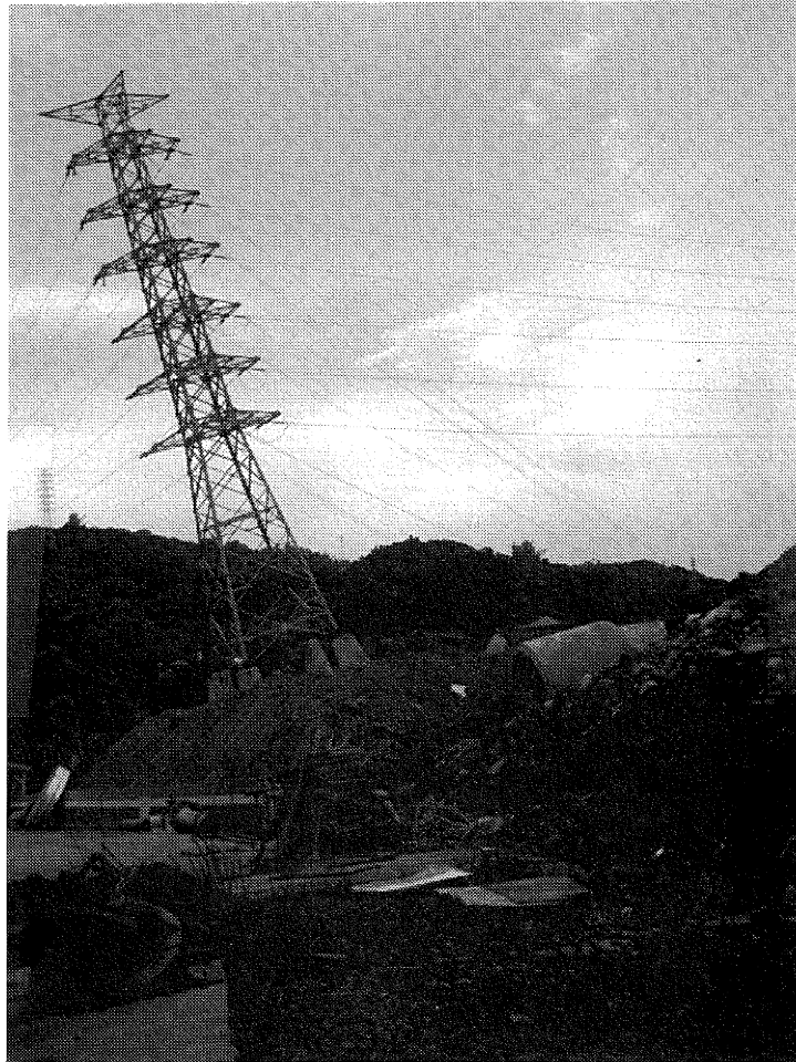
Figure 4.4: Deformation of 69 kV Pylon Due to 2 m Uplift near Mingchien.
