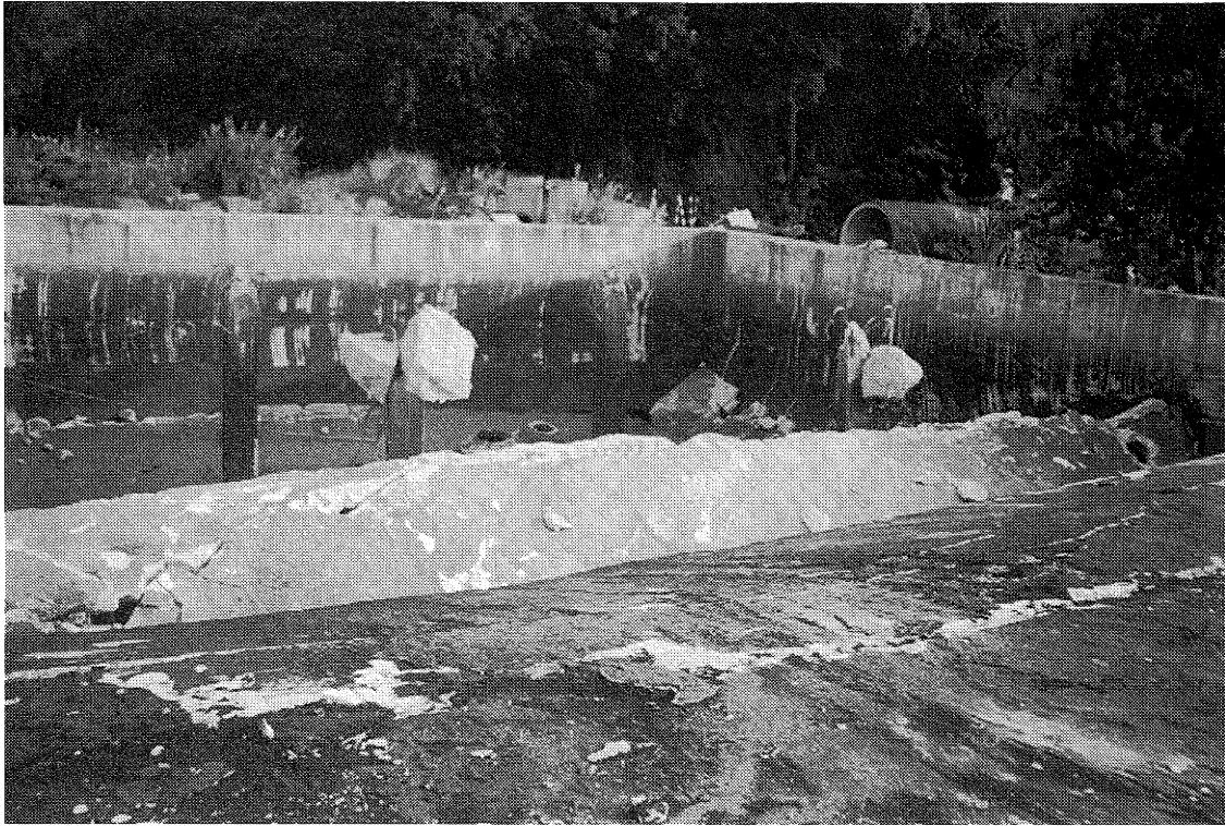
Figure 4.8: Failure of reservoir roof, Fengyuan Water Treatment Plant.
