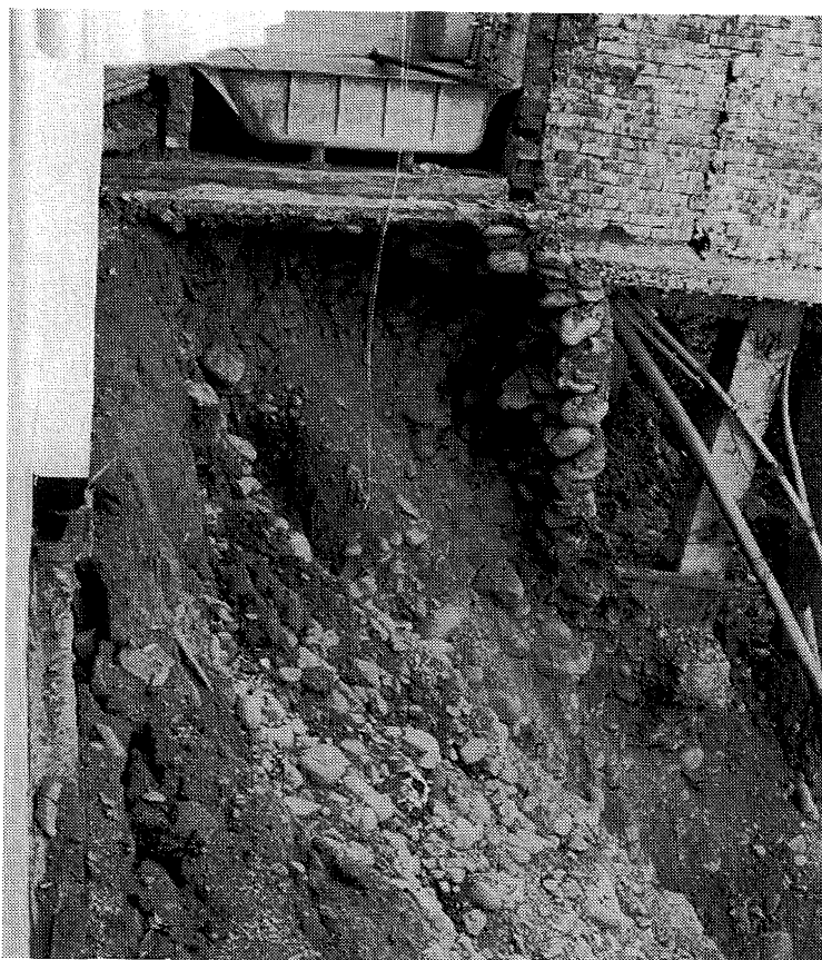
Figure 3.15: Landslide in an elevated quaternary terrace, Chongsing Village.
