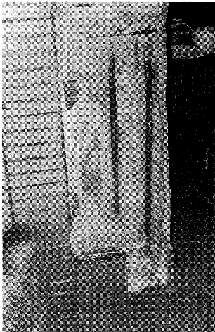
Figure 5.18: Same building as Fig 5.17 showing spalled cover to ground floor column at location of splice to longitudinal bars. Non confining reinforcement to the splice and inadequate cover.
