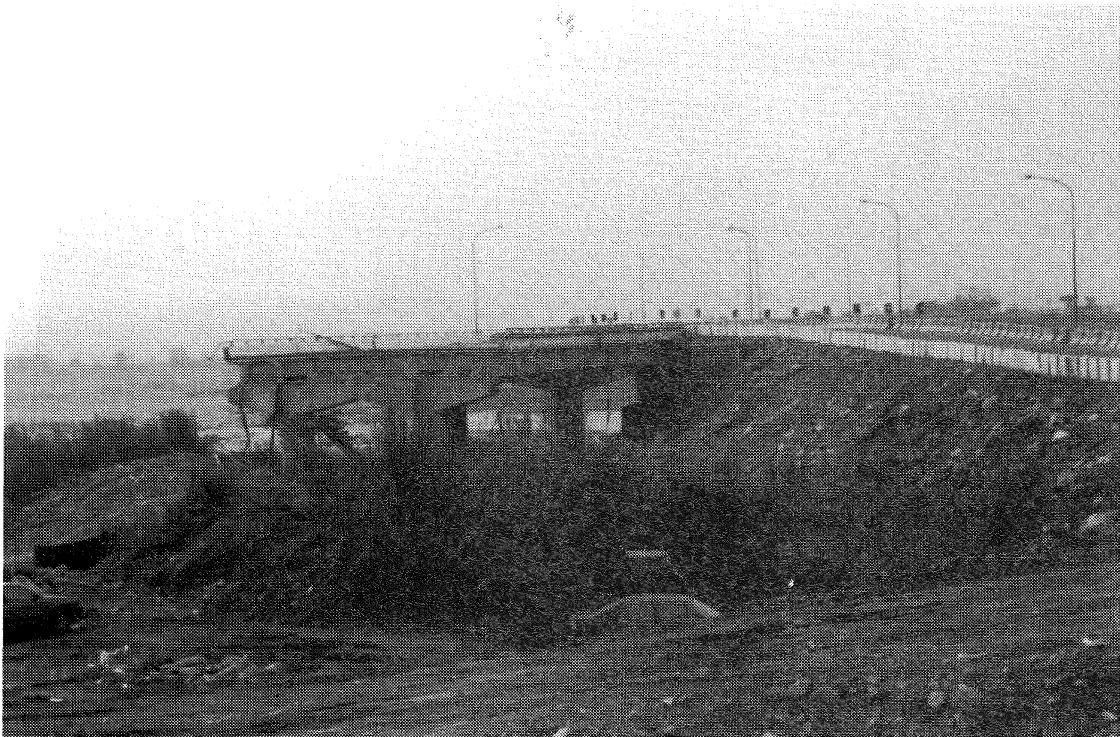
Figure 6.4: Damage to abutment span of bridge crossing the Chosui river.
