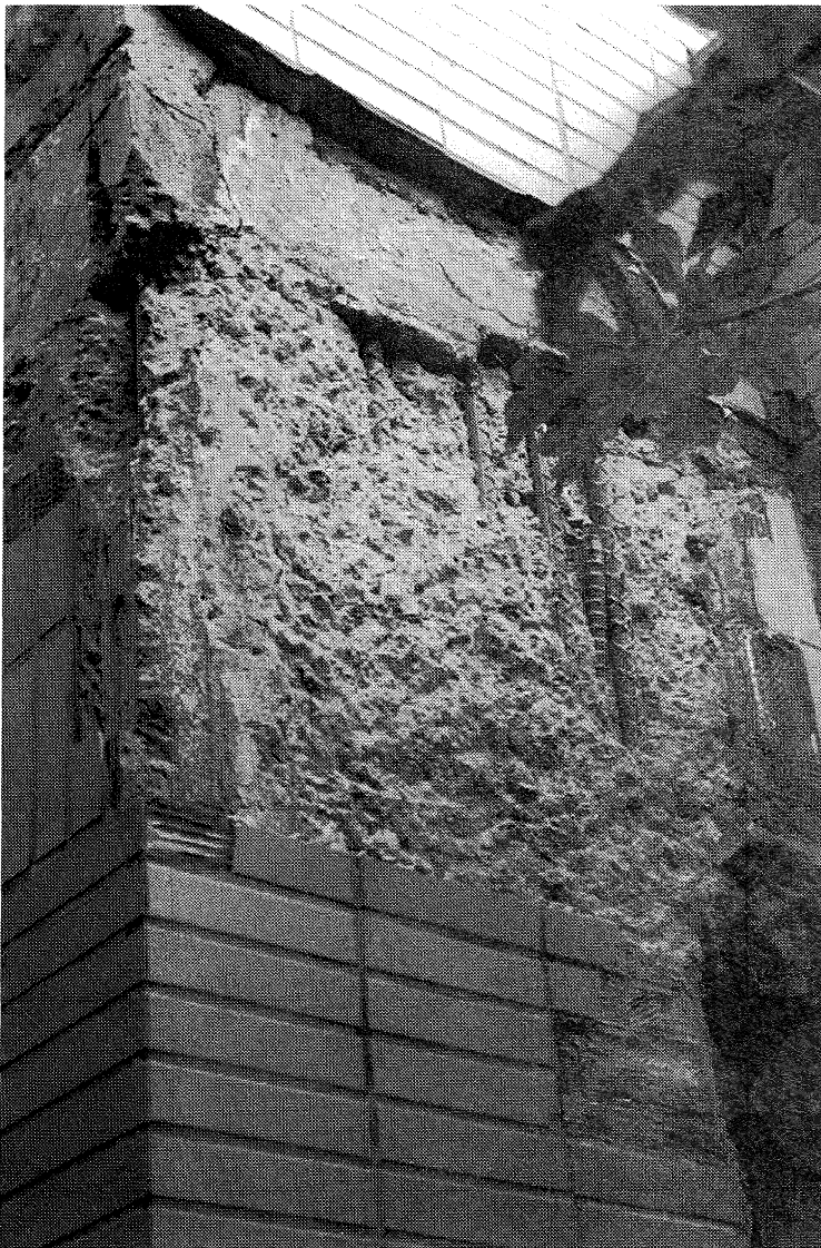
Figure 5.17: Damage to beam corner column junction at first floor level of complex shown in Fig 5.15. Inadequate joint ties and poor quality concrete evident.
