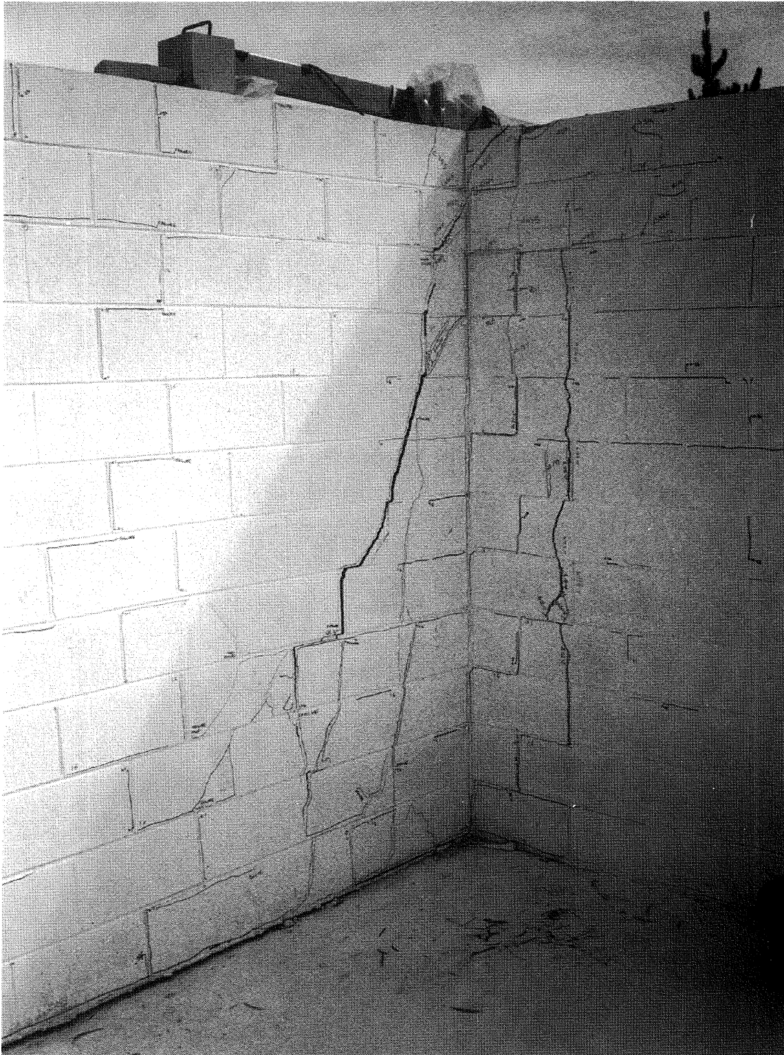
Figure 9: Main wall and return wall B at the end of the test.
