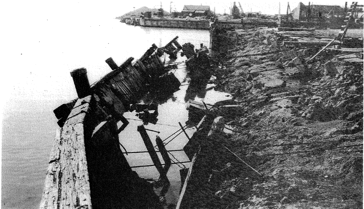
Figure 7: View northwards along failed West Quay at Port Ahuriri, Napier. (Courtesy of the Alexander Turnbull Library, D.H. Jones Collection, Wellington).
