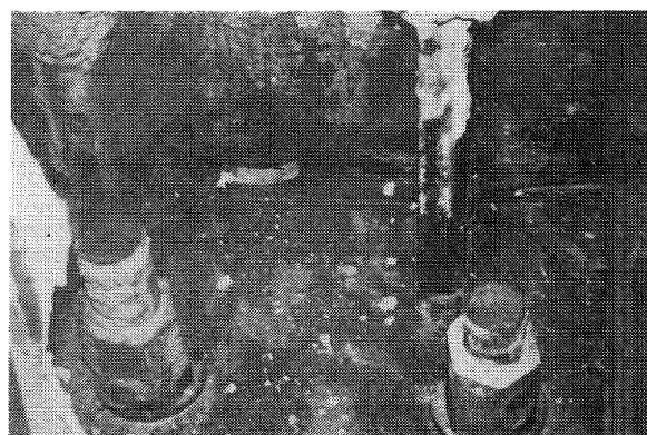
FIGURE 5. Fracture across base plate
