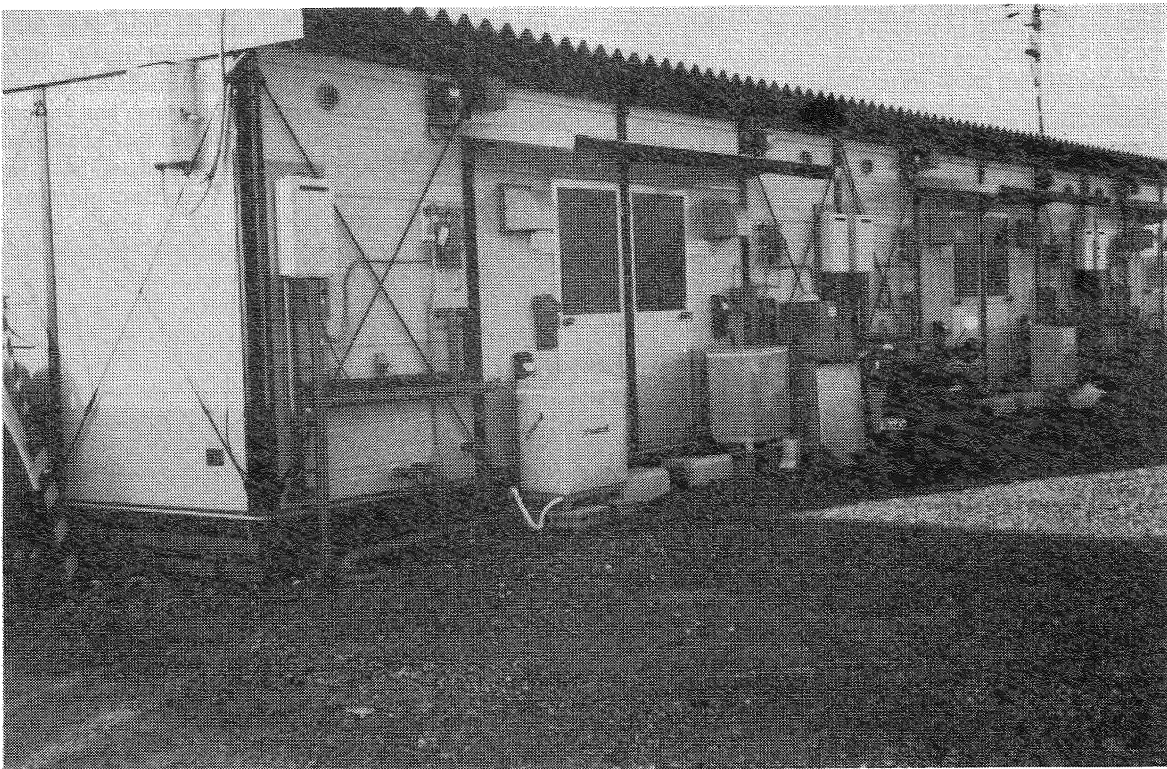
FIGURE 12.2 Temporary Housing Units Showing Services Reticulation
