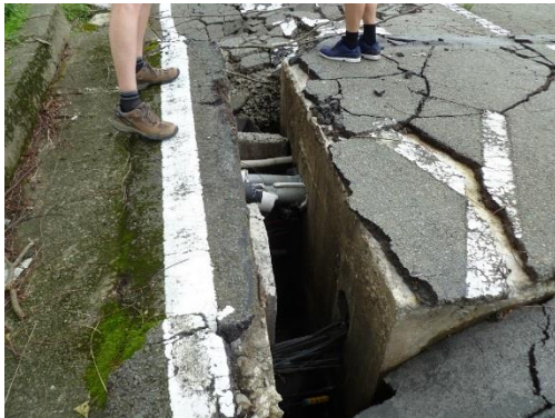
Photos 14 & 15: Ground and underground services disruption Building A13.
