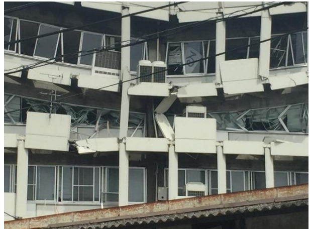
Photo 5: Beam-column joint shear failure and dislocation of beam from column.
