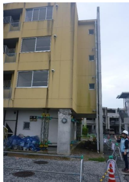
Photo 4: Plastic hinge at top of column.
