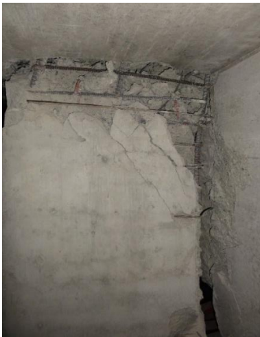
Photo 6: Failure at joint between floor slab & lead dampers.
