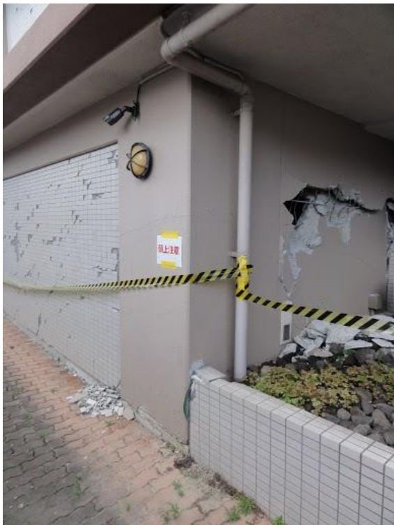
Photo 11: Damaged orthogonal walls at the NE corner (Photo taken from outside the building).
