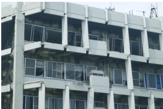
Photo 3: Column plastic-hinge at underside of roof beam and shear failure at Level 4 beam-column joint.
