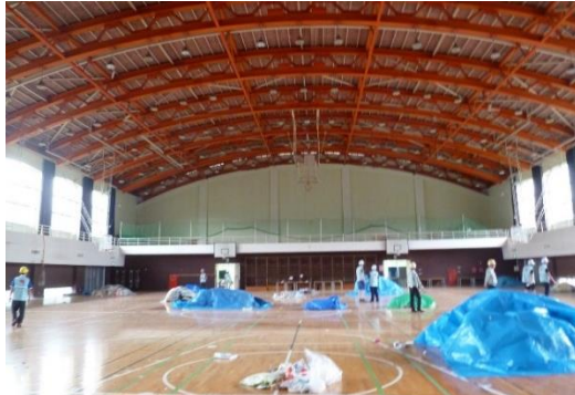
Photo 3: Building interior (note daylight at end wall roof interface).
