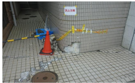
Photo 5: Foundation settlement at base of shear walls due to rocking.
