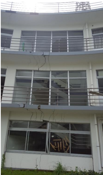
Photos 7, 8 & 9: Visible signs of damage at “Y” juncture of building.
