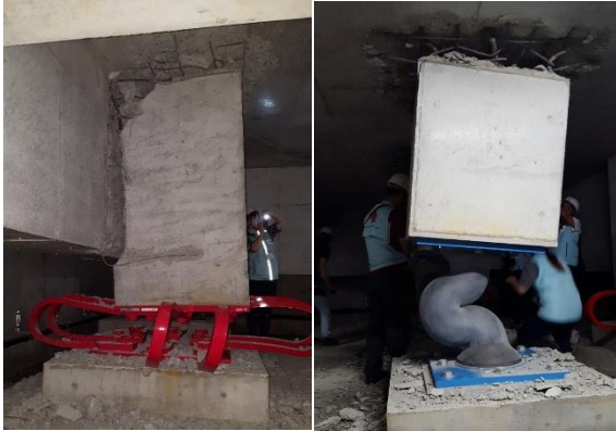
Photos 3 & 4: Separation of steel dampers from concrete beams.
