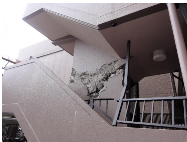
Photo 3: Damage to the first level of stairs on base isolated Building No.2. Staircase isolated at ground level while isolation plane of main structure was at level 1.
