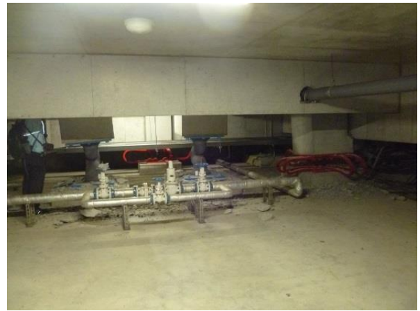
Photo 4: Building A5. Plant and piping in the basement located below the plane of isolation and flexible connectors across the plane of isolation. Note base isolation dampers in background.
