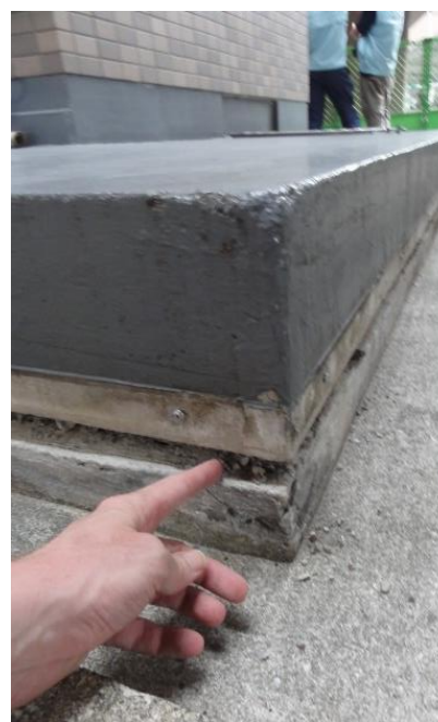
Photo 1: Evidence of residual displacement at base of building
