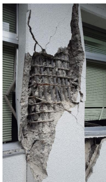
Photo 6: Shear failure of column at centre of building due to short column effect.
