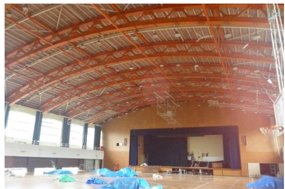
Photo 6: Building A7 designed with no ceiling thus avoiding damage
