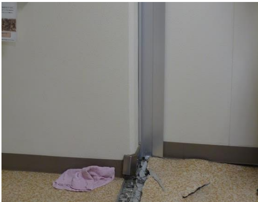
Detail B: Seismic joint between four storey block and interconnector at building interior showing some damage to floor at joint.
