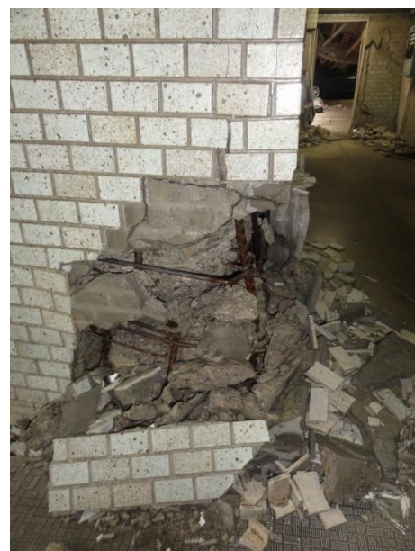
Photo 5a: crushed columns at corners of walls around core.
