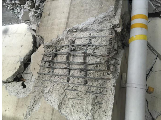
Photos 6 & 7: Close up view of typical columns failed in short column induced shear failure.
