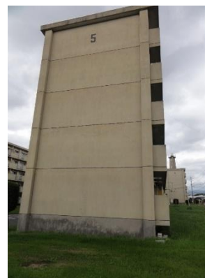
Photo 2: Visible leaning of Building No. 5 (One side noticeably lower than other).
