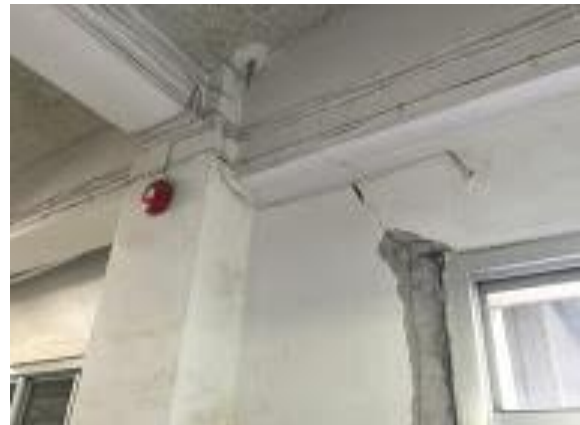
Photo 8: Typical damage to concrete “non-structural” walls between concrete moment frames.
