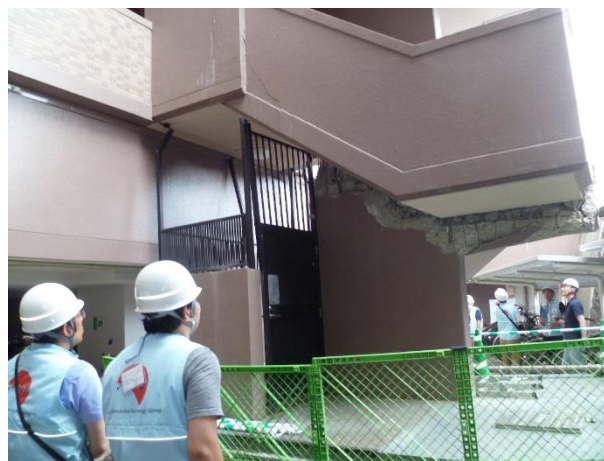
Photo 4: Damage to the first level of stairs on base isolated Building No.2. Staircase isolated at ground level while isolation plane of main structure was at level 1.
