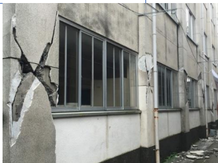
Photo 1: Damaged columns from outside the building
