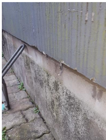
Photo 2: Damage to the first level of stairs on Building No.2 with multi-level isolation
