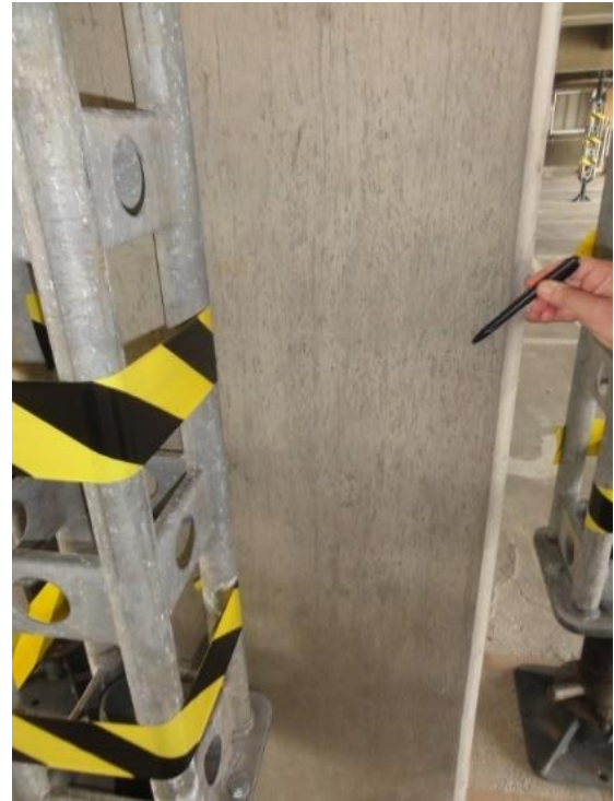
Photo 3b: Apparent torsional cracks.
