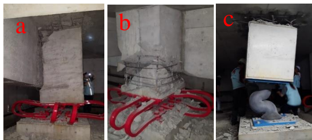
Figure 6: Damage sustained to Steel (a) & (b) and lead (c) dampers below Base Isolated Building No. 1.
