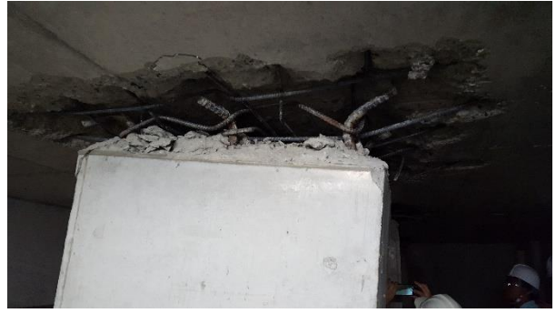
Photo 7: Failure at joint between floor slab & lead dampers.
