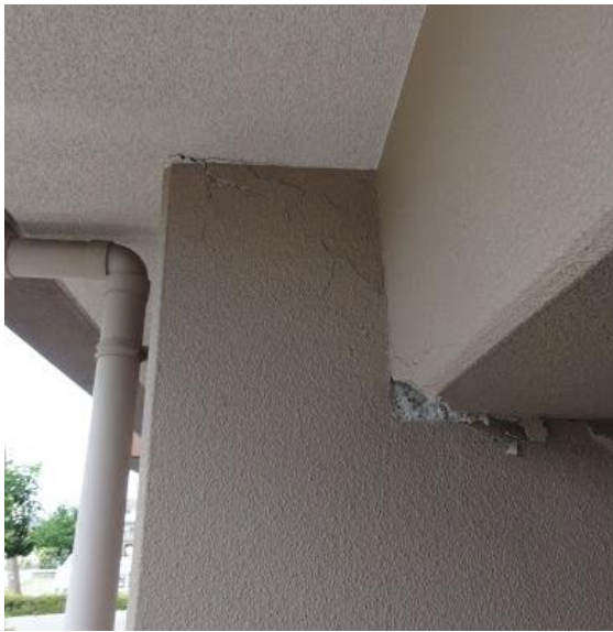
Photo 4: Damage to the central beam-column connection on the south frame.
