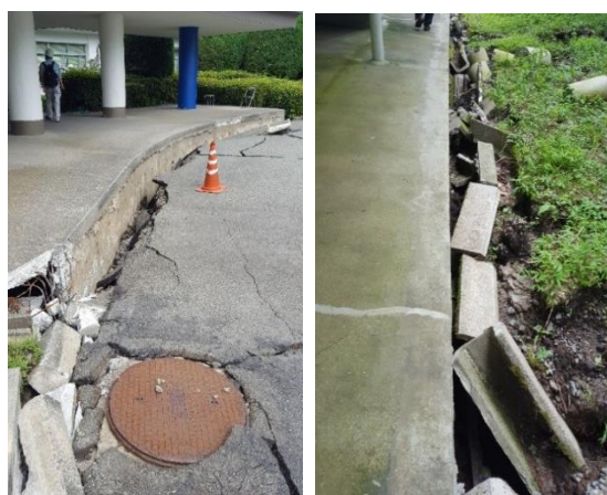
Photos 3 & 4: Ground subsidence around building.
