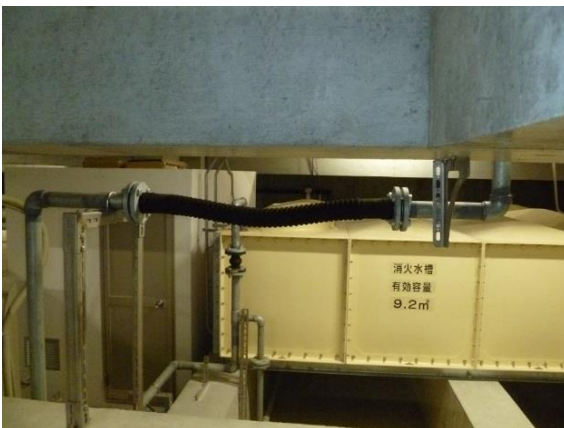
Photo 3: Building A5. Plant and piping in the basement located below the plane of isolation and flexible connectors across the plane of isolation.
