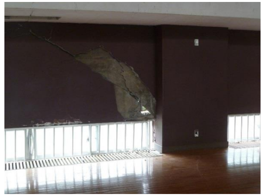
Photo 4: Shear cracking damage to concrete beam supporting mezzanine on side wall.
