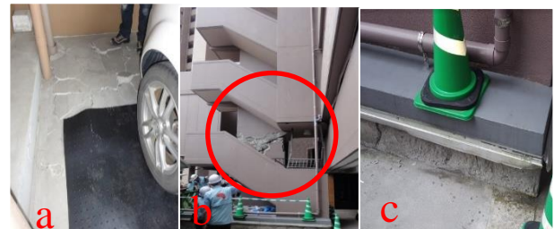
Figure 5: External damage to base isolated buildings (a) Base Isolated Building No.1 (Appendix A5) (b) & (c) Base Isolated Building No.2 (Appendix A6).
