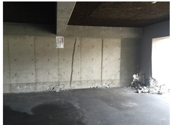
Photo 9: Shear cracks on the east side wall and damage to the south-east corner column.
