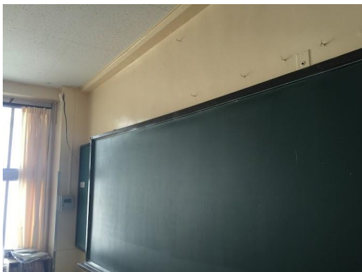
Photo 4: A rare instance of damage to the classroom side external columns.
