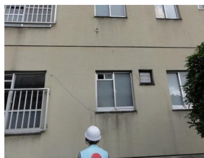
Photo 1: Cracking of non-structural walls due to differential settlement of building.
