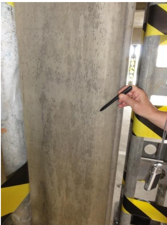
Photo 3a: Apparent torsional cracks.
