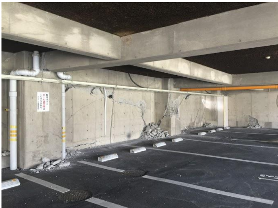
Photo 5: Damaged walls and column on the north side.
