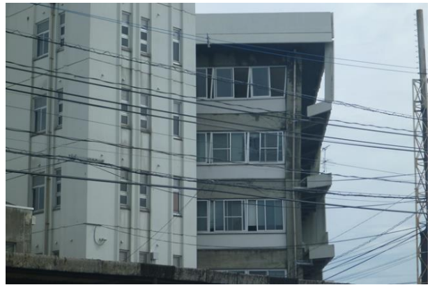
Photo 4: Beam plastic-hinges and permanent offset of upper floors.
