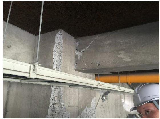
Photo 8: Beam-Column connection at the top of the shear damaged column.
