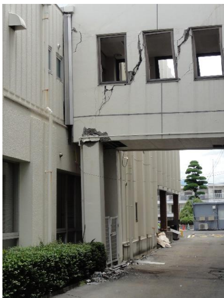
Photo 3: Damage to bridge between two buildings.
