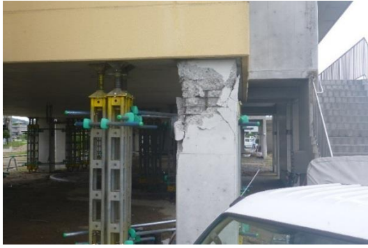
Photo 5: Column plastic hinge with intact concrete core.
