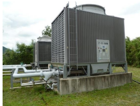
Detail D: Chiller plant located exterior to building. Note ground rupture adjacent to foundations.
