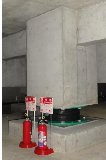
Photo 8: Small base isolator (see floor plan for location).
