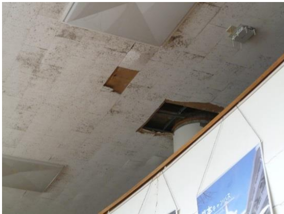
Photo 8: Building A13 interior ceiling damage.
