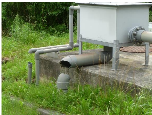
Photo 16: Broken piping adjacent to Building A13.
