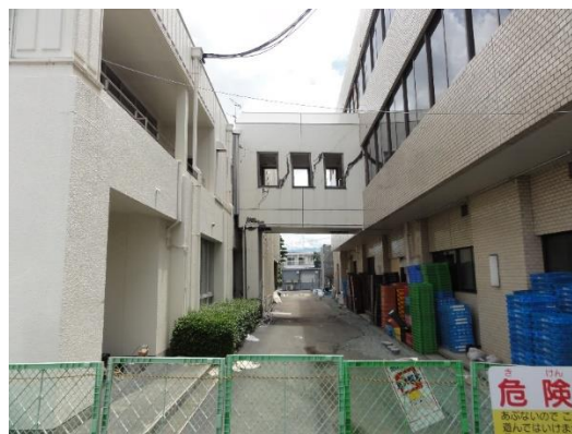
Photo 4: Damage to bridge between two buildings
