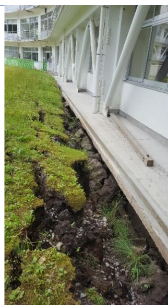
Photo 5: Ground subsidence around building.
