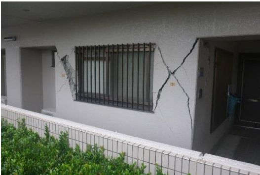
Photo 3: Typical infill concrete wall shear cracking due to interaction with moment frame beams.
