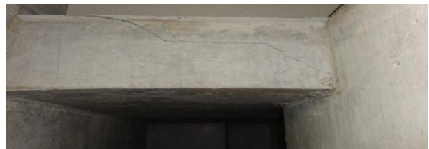
Photo 10: Cracking in deck slab where connected to small base isolator
