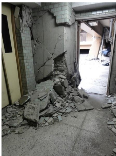
Photo 5b: crushed columns at corners of walls around core.
