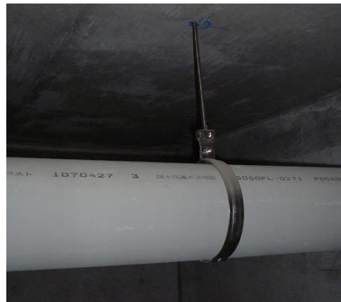
Photo 5: Building A5. Supports for storm water piping located immediately hung from ground floor above the plane of seismic isolation.
