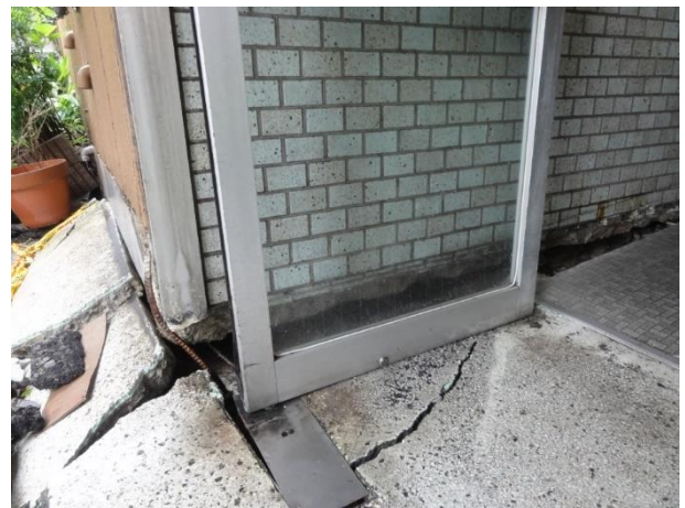
Photo 4: Uplift of wall (does not appear to be structural wall).
