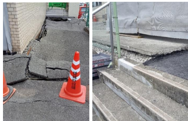
Photos 1 & 2: Ground subsidence around the building.
