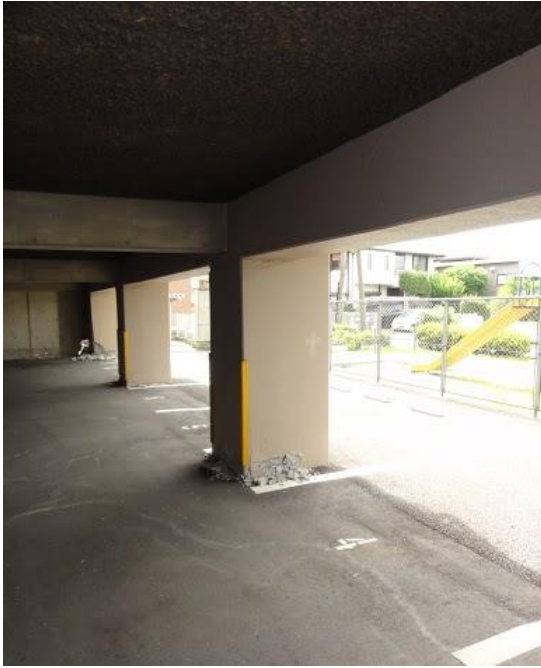
Photo 3: Damage to the columns on South side (most severe damage was to the far-east end column).
