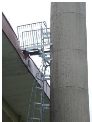
Photos 6 & 7: Chimney adjacent to building (note pounding damage at roof interface).
