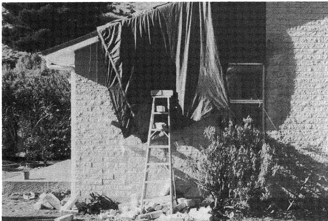
Figure 2. Section of gable end dislodged at the Plant Operators residence, Harpers Village, in the magnitude 5.8 aftershock.
