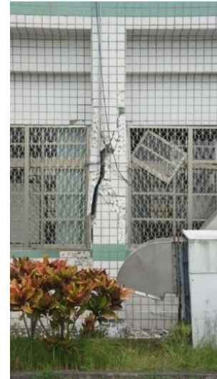
b) Damaged column
