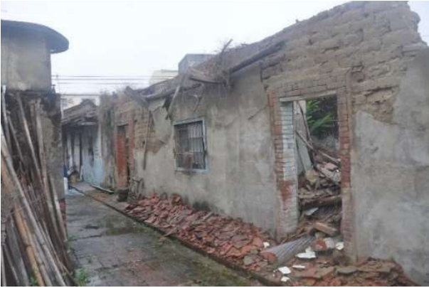
a) Damaged adobe and URM house
