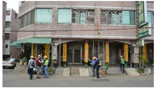
a) Lack of barricading around a red placard building
