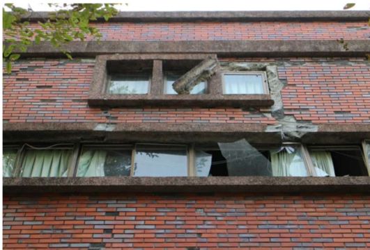
b) Damaged wall
