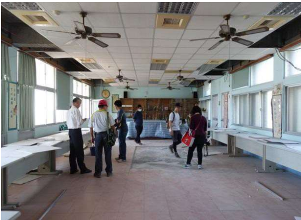
Figure 40: Ceiling tile failure (Source: NCREE).
