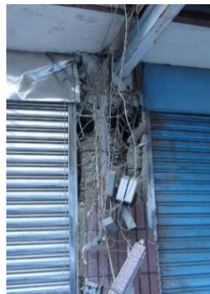
b) Damaged column
