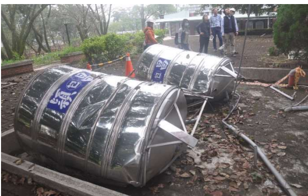
Figure 41: Typical water tanks that were damaged during the earthquake.
