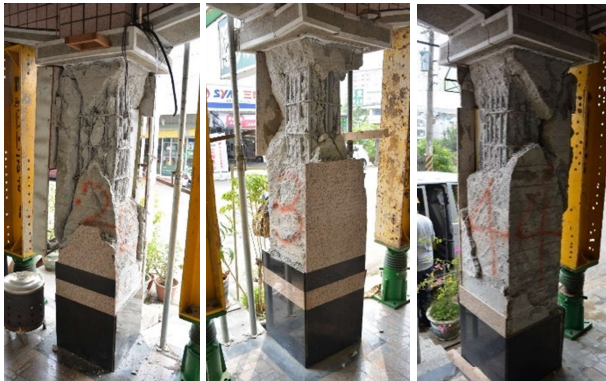
b) Column damage
