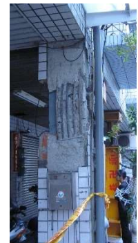
c) Damaged column
