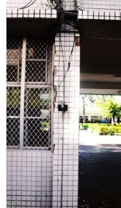
a) Damaged column
