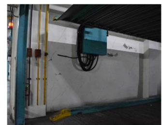
e) Diagonal cracking in wall
