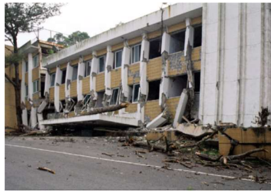
b) Building soft-storey collapse [8]
