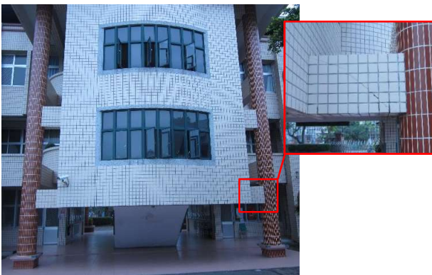
b) Shear crack in support beams
