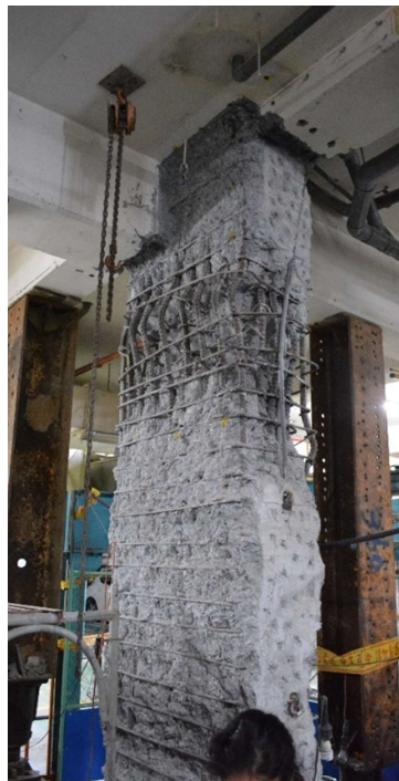
c) Damaged column in basement
