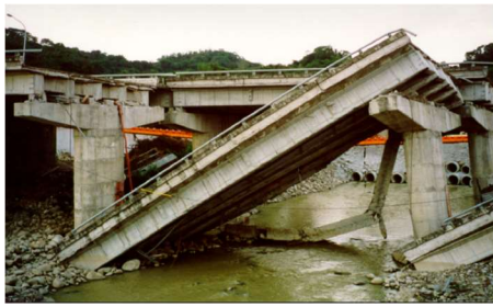
a) Bridge damage [7]
