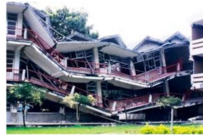
c) School building damage [9]
