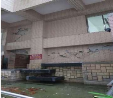
b) Infill wall damage (Source: Prof. Y-H Tu)
