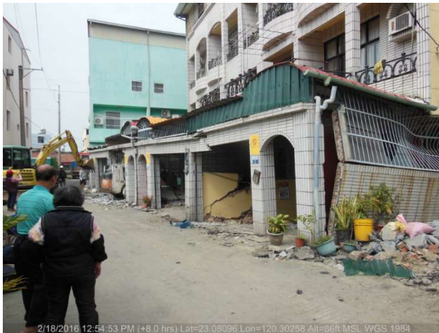
a) Damaged ancillary buildings (GEER [20])
