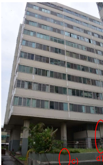
b) Rear view of damage tower
