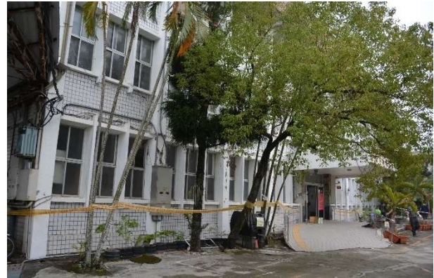
b) Hazard tape surrounding severely damaged building
