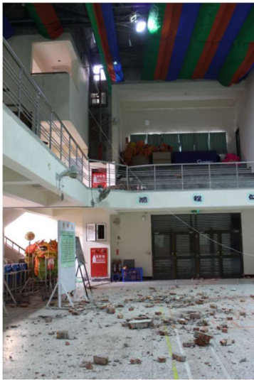
a) Falling bricks inside
