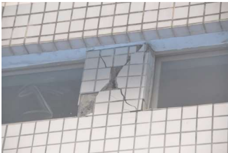
a) Damaged short column
