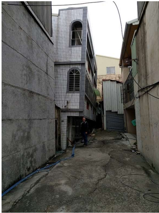
a) Tilted residential building
