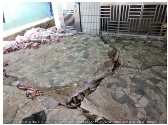
d) Damaged ground slab in front of dwelling (GEER [20])
