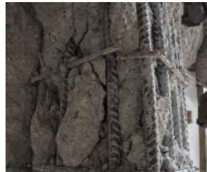
b) Fractured stirrup
