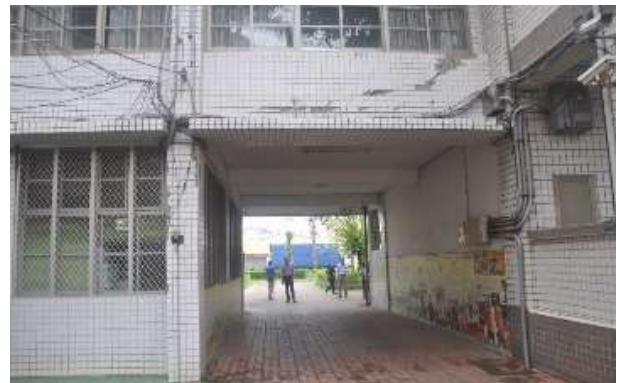
b) Building pounding
