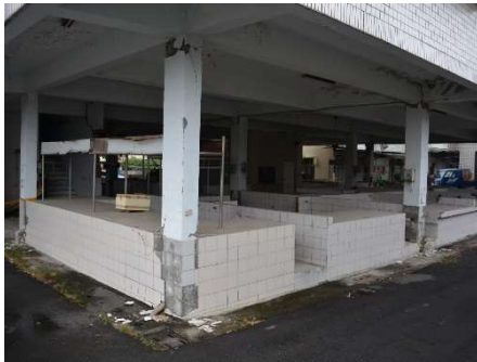
b) Column damage
