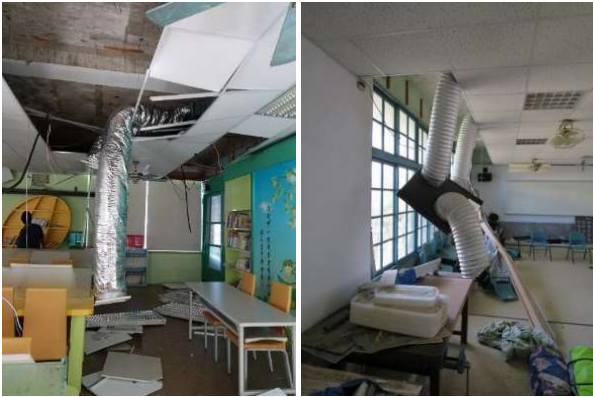
Figure 39: Mechanical ducting support failure (Source: NCREE).
