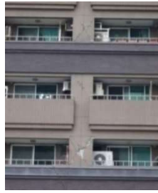
c) Column damage (Source: Prof. Y-H Tu)
