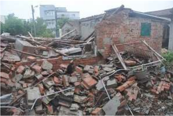
b) Collapsed URM house
