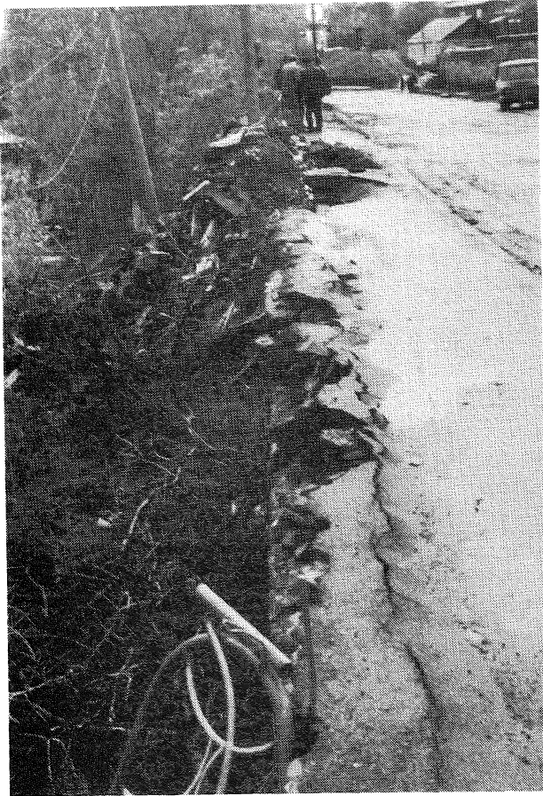
Figure 22 Collapsed wall, Spütak.
