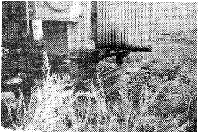
Figure 41 Transformer at Spítak jumped off track.
