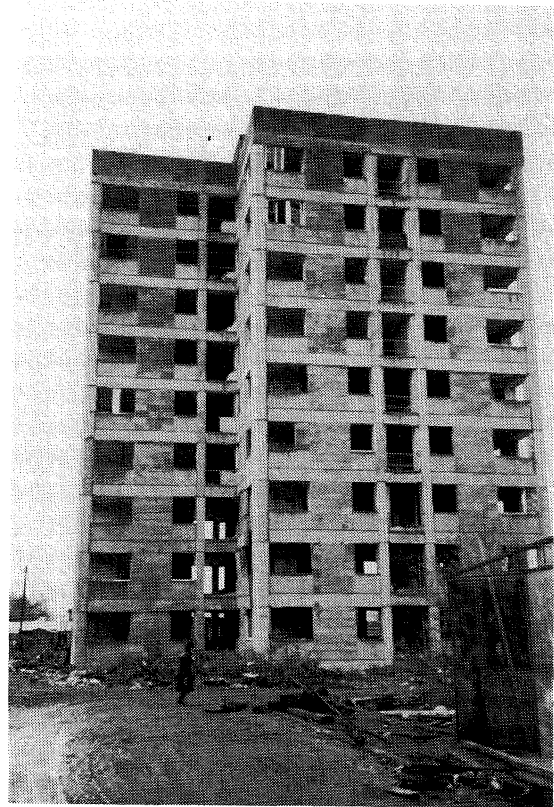
Figure 31 Type 111 building, heavily damaged but still standing, at Leninakan.
