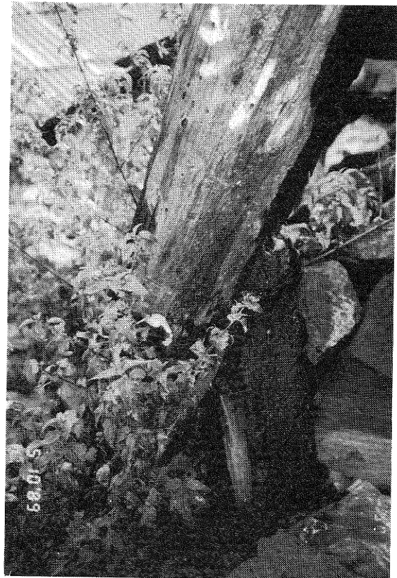
Figure 49 Close up view of power pole fixing failure at Spitak.
