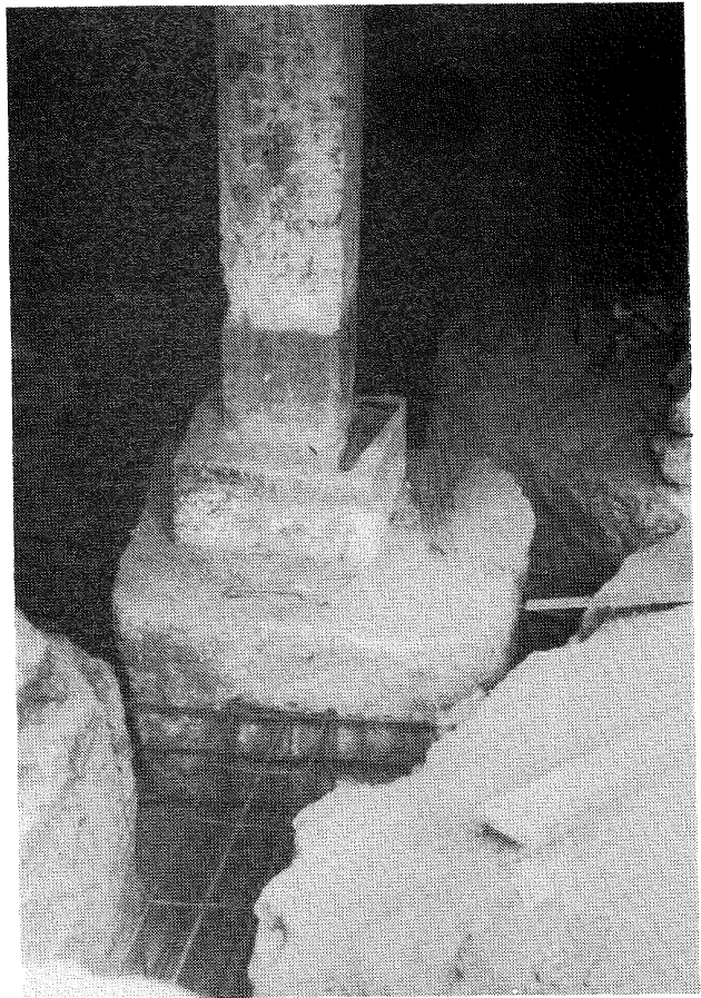
Figure 23 Spread footings being extended and tied together in old quarter of Leninakan.
