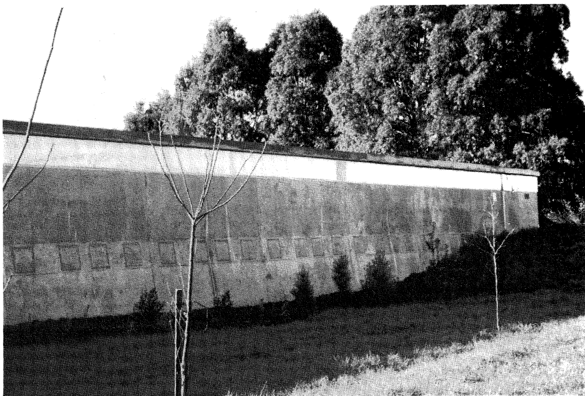
Figure 9 General view of part of the 38,000m 3 water supply reservoir on Hospital Hill, Gisborne. The 140m by 70m reservoir is divided into two cells, and the flashing is in the gap between the external wall and floating slab roof.
