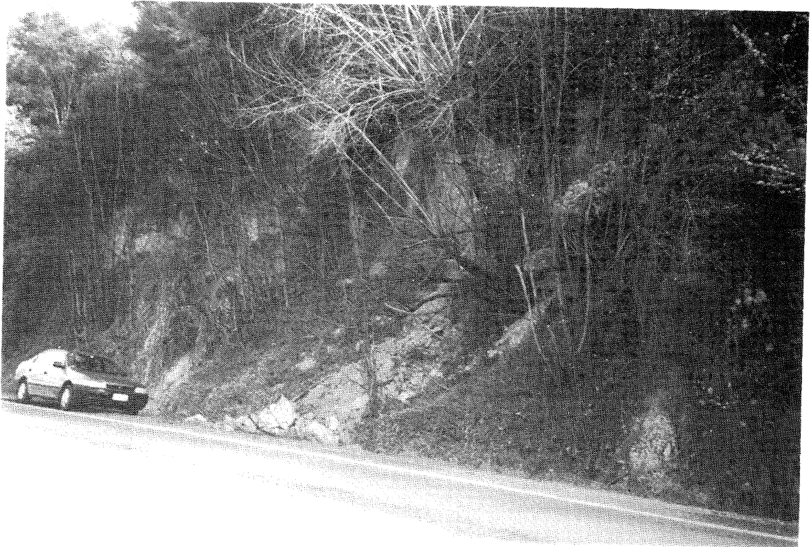
Figure 15 Typical small fall from a steep cut slope beside SH2, 3km north of Kaitaratahi. Fall volumes were typically up to 20m 3 , while other failures which involved bedrock and colluvium were up to 100m 3 .
