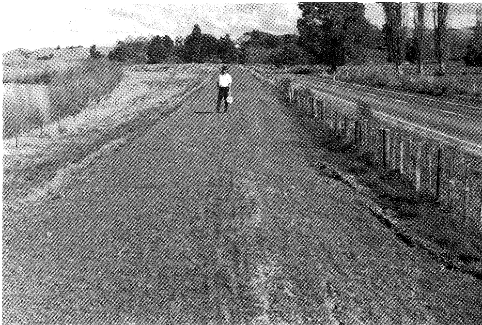
Figure 20 Cracking behind the stopbank on the right (west) bank of Waipaoa River, 2.5km north of Kaitaratahi. Close to a steep bank beside the river, the stopbank has settled by up to 300mm.
