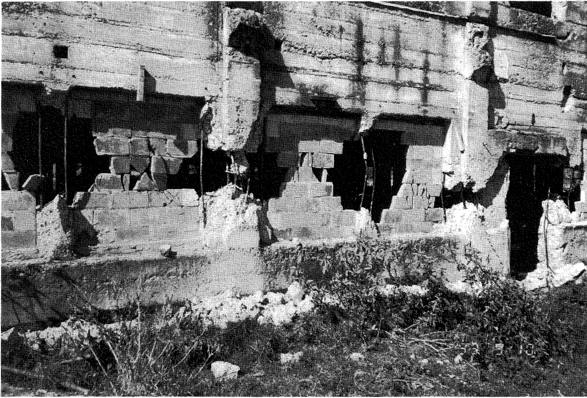
Figure 17 Failure in shear of columns in the southwest wall of the abandoned three-storey freezing works built in about 1915 at Waipaoa. Disused since 1931, only the northwest wall of the building was not damaged.
