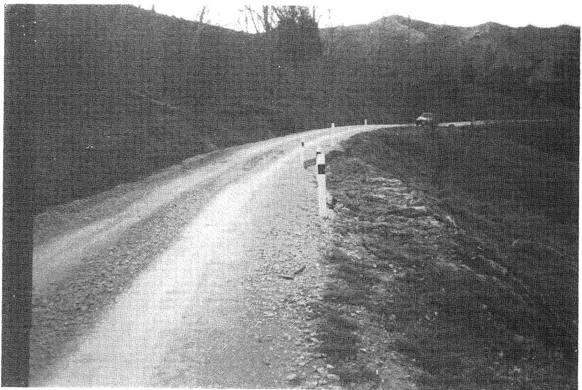
Figure 16 Typical failure involving road surface on Ngakaroa Road, 5km east of Kaitaratahi. Slumping typically occurred on slopes between 15° and 20°, where there was either a veneer of colluvium above bedrock or fill materials.
