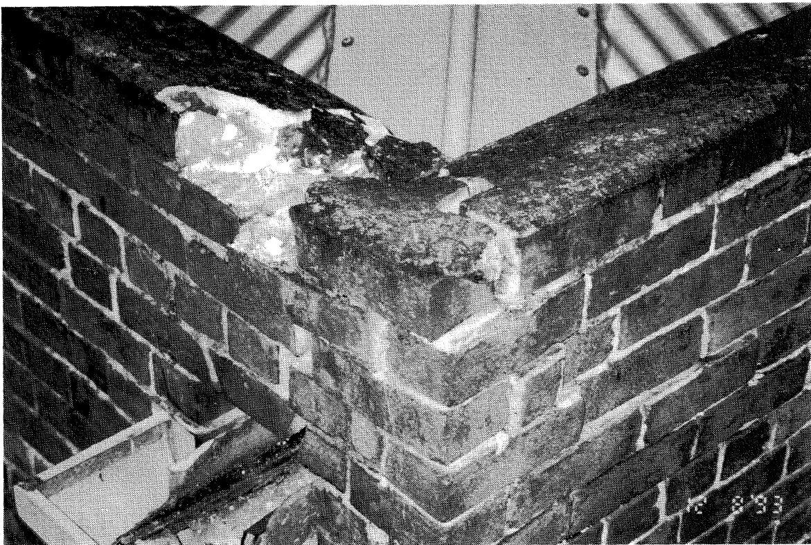
Figure 6 Close up view of cracking in parapet corner of the building in Figure 5.
