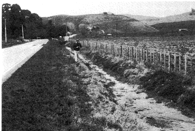
Figure 27 Boils (#101 and #103) in drain beside the road at Site 4.
