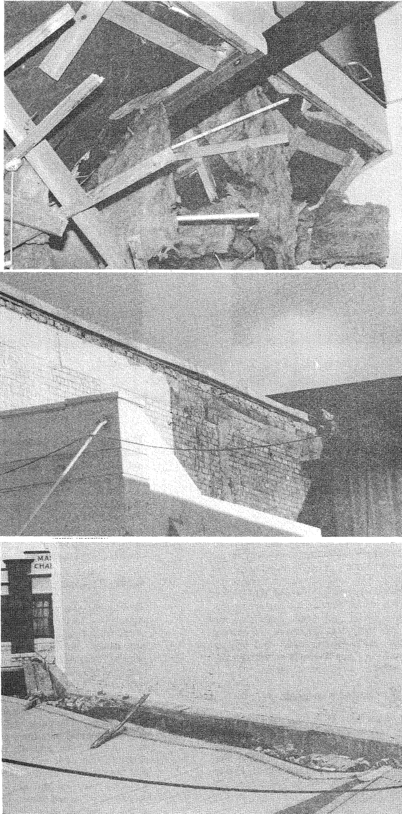
Figure 7 Damage to the Trustbank building.
