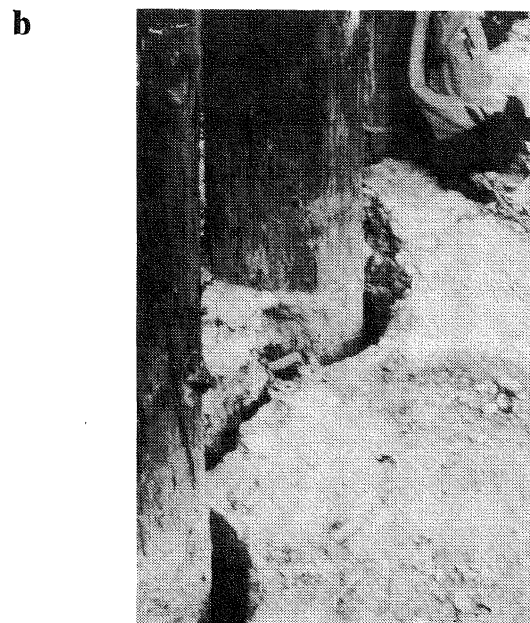
Fig. 2.8 Gapping after the Loma Prieta earthquake: (a) adjacent to a 2 m diameter bridge pier, and (b) adjacent to timber piles at the foundations of a railway bridge near Watsonville.
