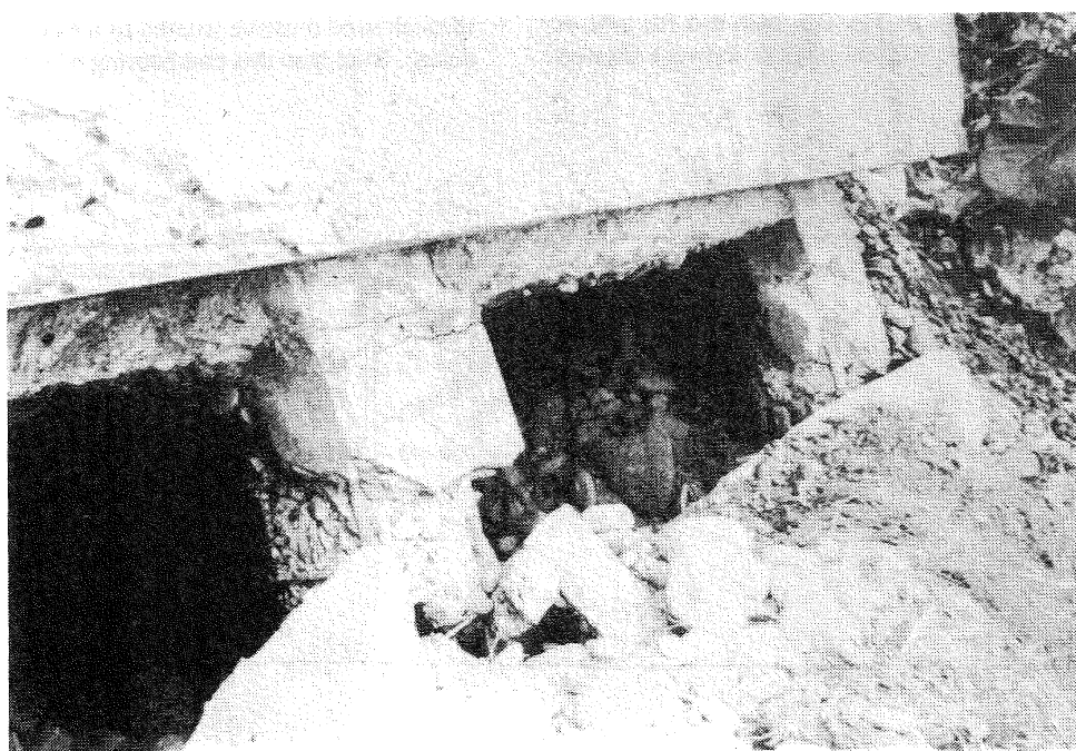
Fig. 2.5 Damage to the raked piles of the Rio Banano bridge abutment during the 1991 Costa Rican earthquake (after Priestley et al (1991)).
