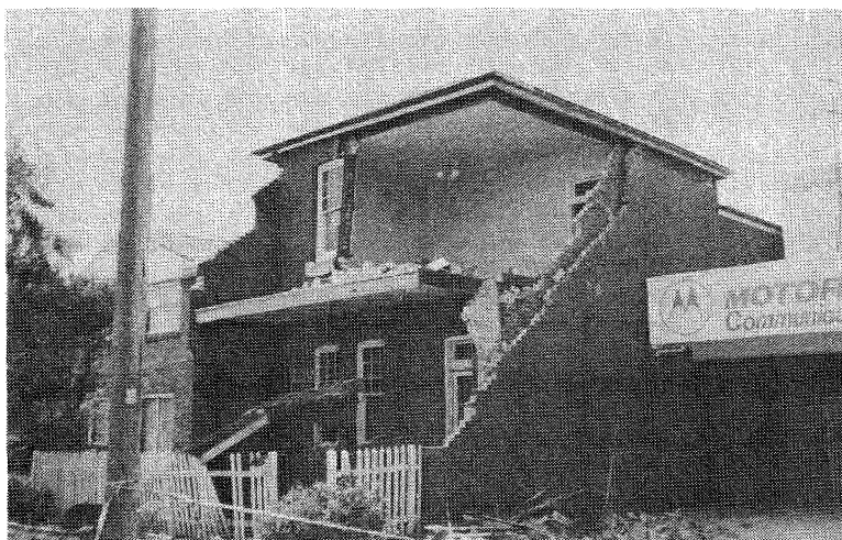
FIGURE 43 TWO-STOREY PRIVATE DWELLING, 49 DENISON STREET, HAMILTON: FAILURE OF CAVITY BRICK WALL WITH NO LATERAL SUPPORT - INTERESTING CANTILEVER ROOF REMAINING (5.1.90; C.R. FEATHERSTONE)
