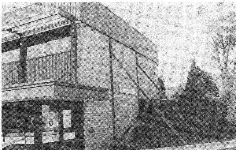
FIGURE 29 ROAD TRAFFIC AUTHORITY BUILDING, PACIFIC HIGHWAY, CHARLESTOWN: SHORING OF UNREINFORCED CAVITY MASONRY FEATURE END WALL WHICH WAS NOT TIED LATERALLY TO AND BECAME SEPARATED FROM SIDE WALLS (20.1.90; E. BRENNAN)
