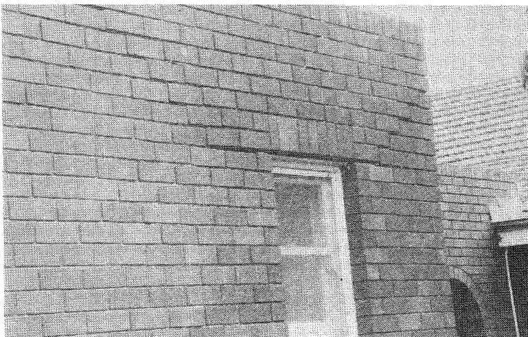
FIGURE 10 LIVERPOOL CHILDREN'S HOSPITAL, SYDNEY, 150 km SW OF NEWCASTLE: TYPICAL MASONRY DIAGONAL SHEAR FAILURE FROM WINDOW LINTEL (22.1.90; E. BRENNAN)
