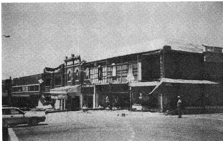
FIGURE 36 COMMERCIAL BUILDINGS, KING AND UNION STREETS, NEWCASTLE CBD: OUTER SKIN OF BRICKWORK COLLAPSED ONTO AWNING - INSIDE TIMBER FRAME SUPPORTING ROOF REMAINED IN PLACE (29.12.89; J.M.W. RYNN)
