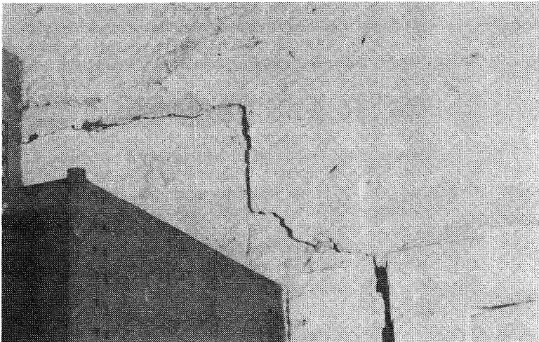
FIGURE 32 NORAH HEAD LIGHTHOUSE, OPERATIONS ROOM: MASONRY SHEAR FAILURE IN CONCRETE BLOCK WALLS WITH CRACKING AROUND CONCRETE MAIN FRAME (20.1.90; E. BRENNAN)
