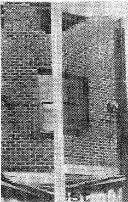
FIGURE 75 BLOW-UP OF FIGURE 38 (BUILDING IN BEAUMONT STREET, HAMILTON) TO SHOW TYPICAL FAILURE OF AWNINGS IN MANY PARTS OF NEWCASTLE WHERE IN EITHER AWNING TIE RODS BROKEN BUT STILL CONNECTED IN PART TO MASONRY WALL SUPPORTS (RHS) OR PULLED OUT OF WALL SUPPORTS (LHS) (4.1.90; C.R.FEATHERSTONE)
