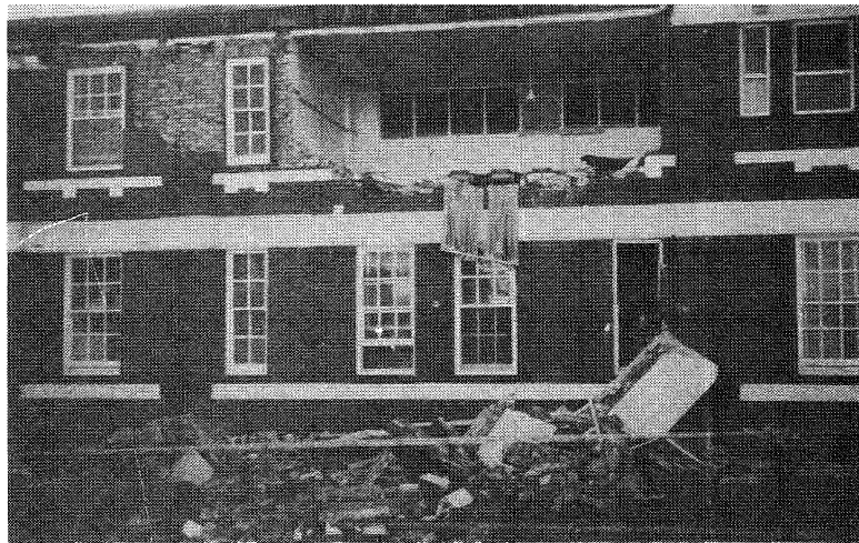
FIGURE 26 HAMILTON AMBULANCE STATION (REGIONAL HEADQUARTERS), DENISON STREET AND PARKWAY AVENUE, HAMILTON: MASONRY FAILURE OF BOTH SKINS DUE TO LACK OF LATERAL SUPPORT WALLS. BUILDING ALSO SUFFERED OTHER SEVERE MASONRY DAMAGE (29.12.89; J.M.W. RYNN)
