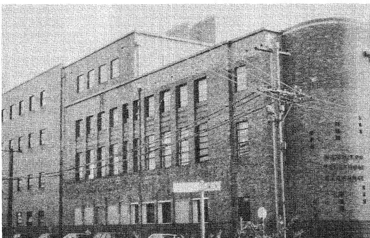
FIGURE 30 TELECOM TELEPHONE EXCHANGE, DENISON AND LAWSON STREETS, HAMILTON: REPAIRED DAMAGE TO UNREINFORCED MASONRY LOADBEARING WALLS OF BRICKWORK SEPARATION AT DISCONTINUITIES IN UPPER PARTS OF OLDER SECTION AT FRONT (21.3.92; D.J. WILLIAMS)
