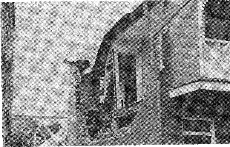
FIGURE 41 TERRACE HOUSE, LAMAN STREET, COOKS HILL: COLLAPSE OF DOUBLE SKIN BRICK WALL AND BRICK GABLE END WITH NO LATERAL SUPPORT OF TWO-STOREY PRIVATE DWELLING, TYPICAL DAMAGE FOR THIS TYPE OF CONSTRUCTION (5.1.90; C.R. FEATHERSTONE)
