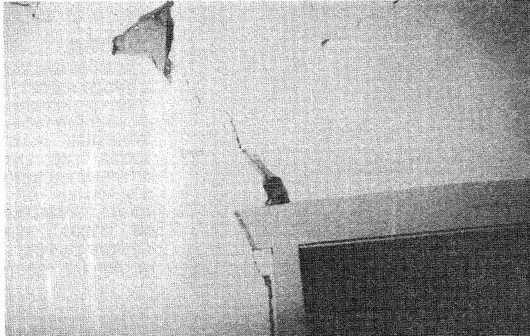
FIGURE 44 INTERIOR OF SINGLE STOREY PRIVATE DWELLING, 91 MEREWETHER STREET, MEREWETHER: TYPICAL DIAGONAL SHEAR FAILURE IN UNREINFORCED MASONRY WALLS (BRICK AND CEMENT RENDER) FROM DOOR OPENING IN INTERNAL WALL SHEETING (4.1.90; B. GREEN)
