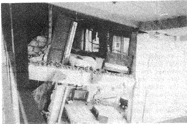
(c) Failure of Masonry Infill Walls.
