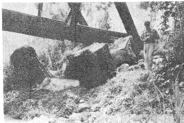
(c) Caissons Rotated Towards River with Support Block Fallen off and behind. (North abutment).
