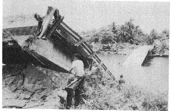
(b) General View showing North Abutment Damage.
