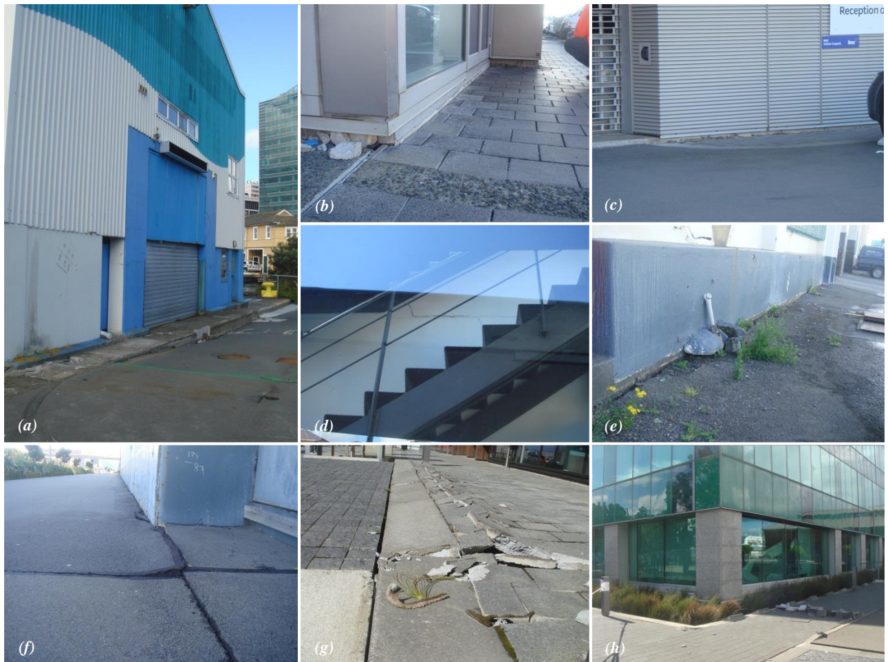
Figure 8: Various states of ground adjacent to structures: (a) ground settlement near a wharf shed; (b) settlement of the ground adjacent to BNZ building; (c) another section of BNZ building showing differential settlement between ground and structure; (d) non-structural damage to the interior of the BNZ building; (e) settlement of ground adjacent to the Customhouse building, resulting in vertical and horizontal offset; (f) cracked pavement and ground settlement near Customhouse building; (g) damaged brick pavement between Customhouse and Statistics NZ building; (h) destroyed pavement in front of Statistics NZ building.
