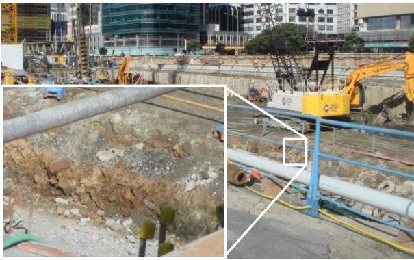
Figure 3: An excavation site at the waterfront for a building, showing the exposed gravel fill.
