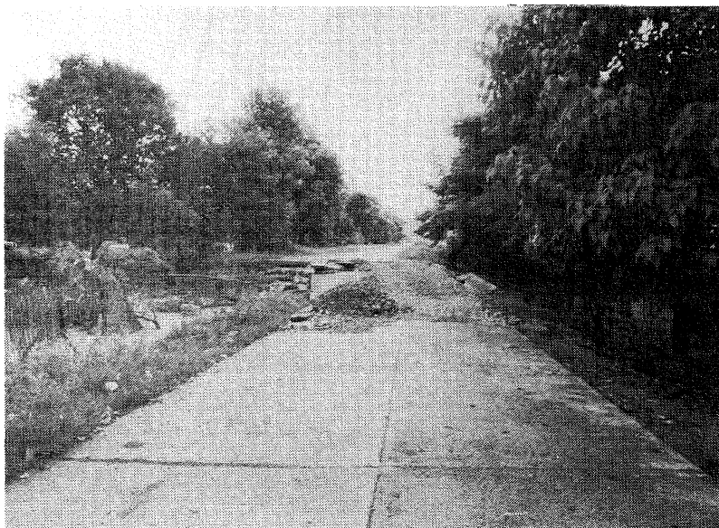
Figure 4.3: From the ground, both the 3 m left lateral, 1.5 m vertical displacement are obvious, as is the damage to the road (Photo: Dodong Teves, PNOC)
