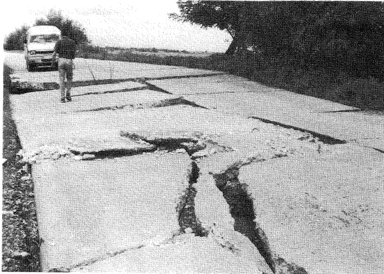
Figure 5.1.14: Liquefaction in low lying alluvial areas distorting road fills and pavement surface
