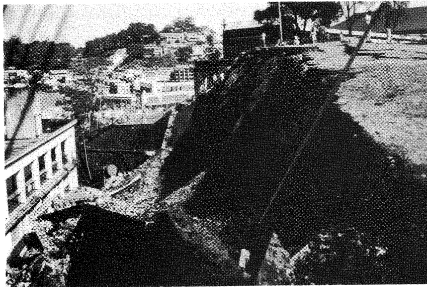
Figure 5.1.22: St Mary's Cathedral, Baguio; approximately 18 m high bank of volcanic pyroclastic material faced with cemented rock and concrete panels
