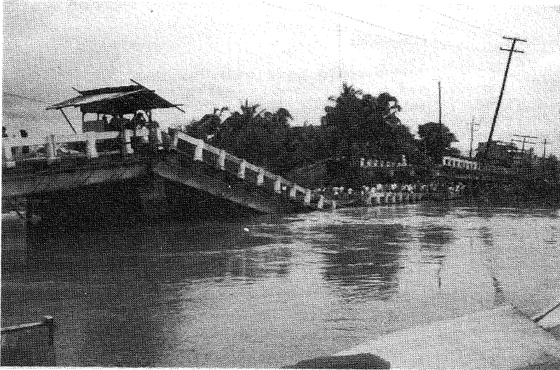
Figure C7.1: Dagupan City, Magaysay Bridge on Perez Blvd.; collapse of bridge spans due to liquefaction and lateral spread of river bank
