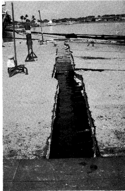
Figure 5.2.12: San Fernando port; tension failure of pier deck
