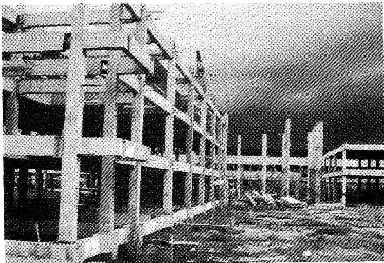
Figure 5.3.19: Precast building under construction near Tarlac. Site connections relied on the welding of large reinforcing bars
