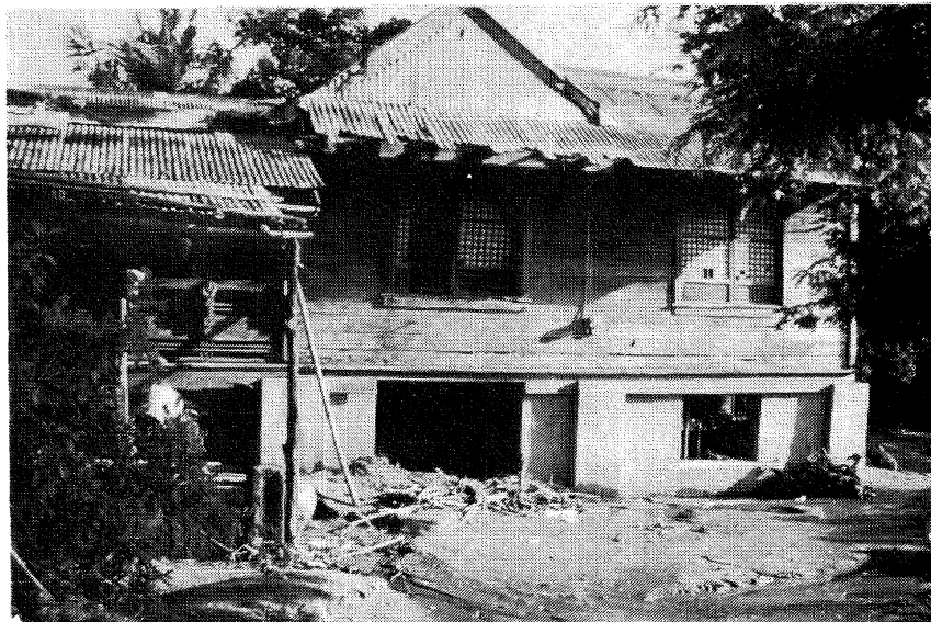
Figure 5.1.9: Settlement of house at Aringay due to liquefaction of foundation soils. The house has settled approximately 1 metre
