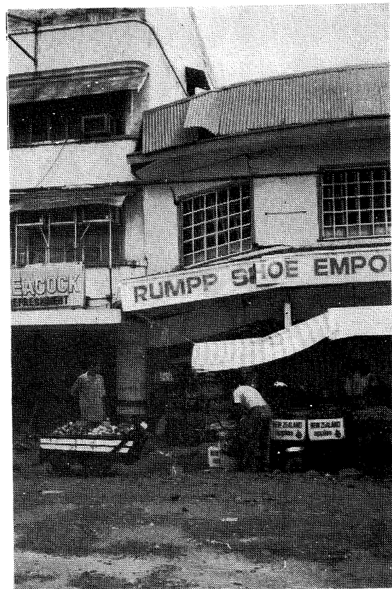
Figure 5.1.8: Dagupan City, A.B. Fernandez Ave, relative settlement of building with different bearing stress
