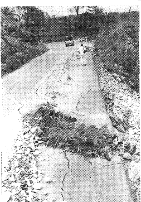
Figure 5.1.21: Road slumping due to failure of rock facing to retain fill
