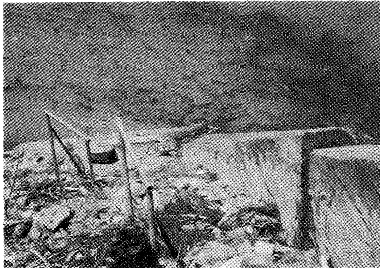
Figure C4.4: Ambuklao Hydroelectric Plant - tilting and separation of spillway wing wall segments due to settlement of rockfill dam
