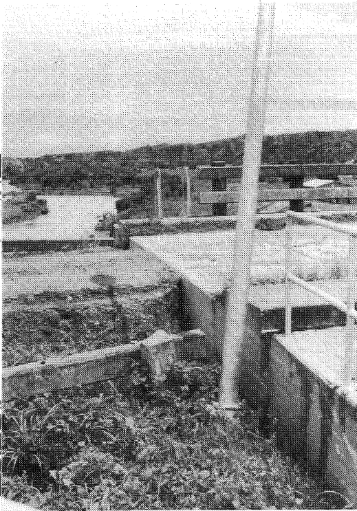
Figure 5.1.24: Masiway Dam; settlement of rockfill dam at spillway interface. Note temporary approach fill
