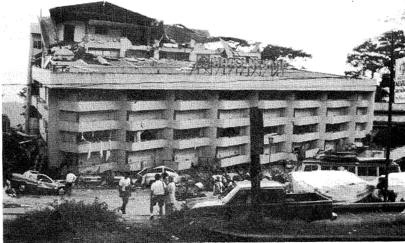
Figure 5.3.1: Effects of soft storey at Hotel Nevada, Baguio
