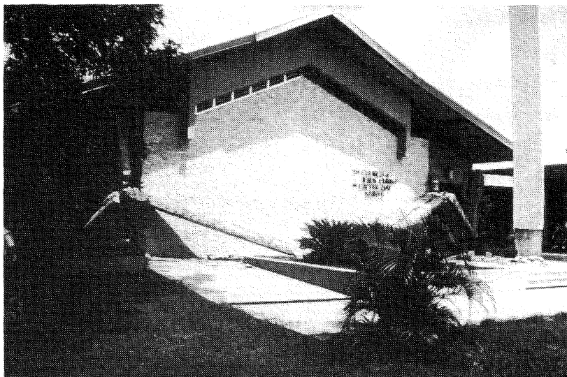
Figure C3.3: Church at Munoz; collapse of reinforced concrete barge board
