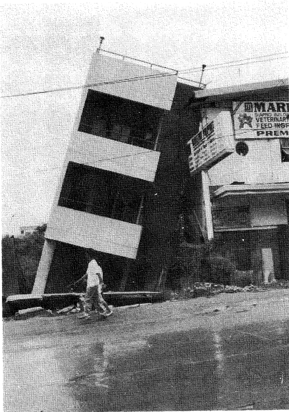
Figure 5.1.7: Dagupan City, Perez Blvd, 3 storey building tilted and impacted on adjacent building
