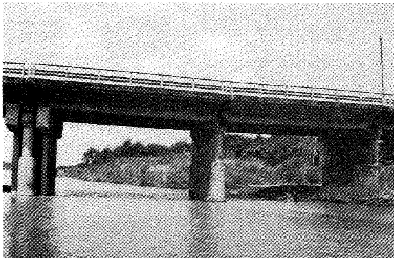
Figure 5.1.10: Binalonan Bridge, settlement of central pier by approximately 0.3 metre. Note previous work to pier on left
