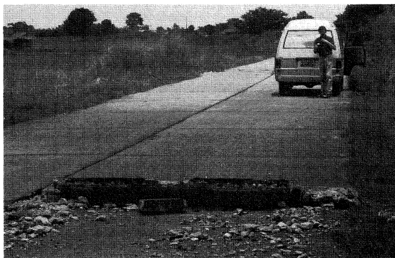
Figure 5.2.2: West of Rizal; compression failure of concrete road paving, typical offset of failure in each carriageway
