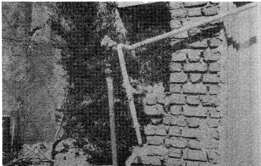
FIGURE 37: DAMAGE TO A GAS PIPE IN A BUILDING IN MANJIL.
