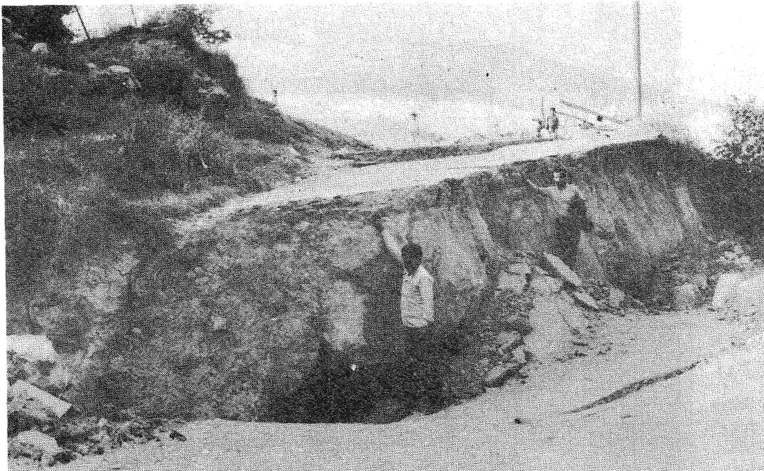
FIGURE 8: VERTICAL DISPLACEMENT CAUSED BY A LANDSLIDE ON THE ROAD TO JIRANDEH IN THE VICINITY OF THE FAULT BREAK.
