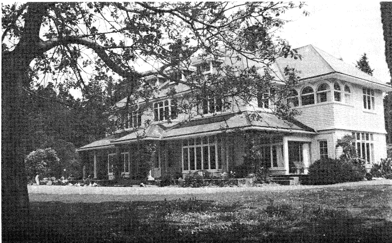
FIGURE 4. THE HOMESTEAD AT SNOWDON. CHIMNEYS FELL, AND THE ORNAMENTAL COLUMNS OF THE VERANDA WERE RACKED SIDWAYS, BUT THERE WAS LITTLE STRUCTURAL DAMAGE.
