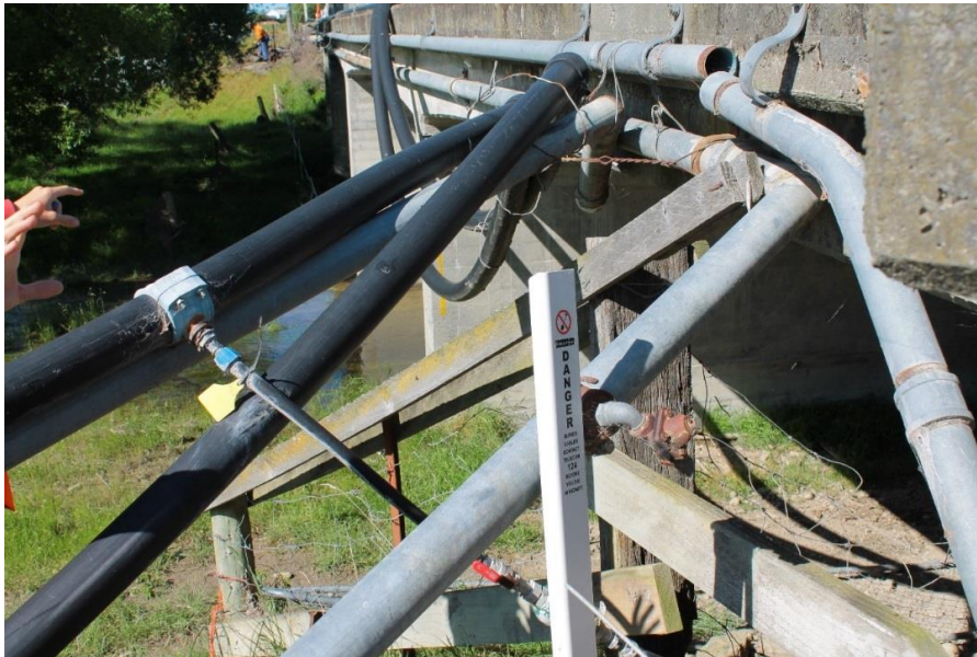
Figure 7. East side of the Needles Creek Bridge north of Ward on the SH1, viewed from the north. Original freshwater pipelines have failed and been replaced temporarily with ductile pipes (in black) (Photo: X. Bellagamba).
