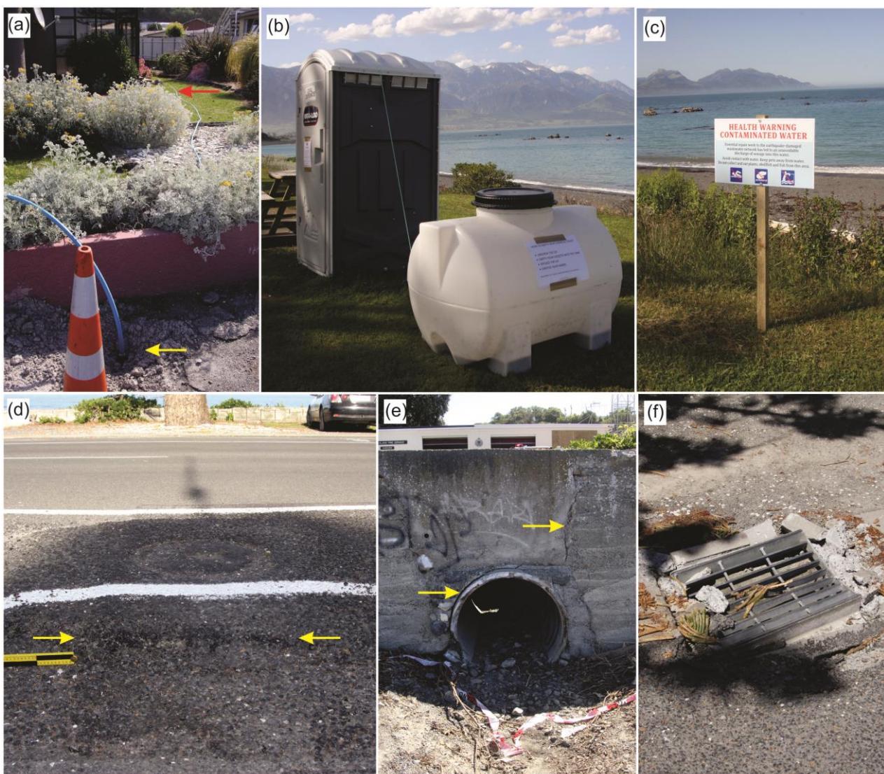
Figure 9. Three waters impacts along The Esplanade, Kaikōura. (a) Temporary overlanding of domestic water supply from the street connection (yellow arrow) to the house's kitchen area (red arrow). (b) Portaloos (left) and chemical toilet dump station (right). (c) Contaminated water warning, discouraging swimming, fishing and shellfish collection. (d) Differential manhole movement of ~3 cm (arrows). (e) Cracking in retaining wall (arrows) surrounding stormwater culvert. (f) Damaged concrete gutter due to impact by steel stormwater grate. (Photos: M.W. Hughes).
