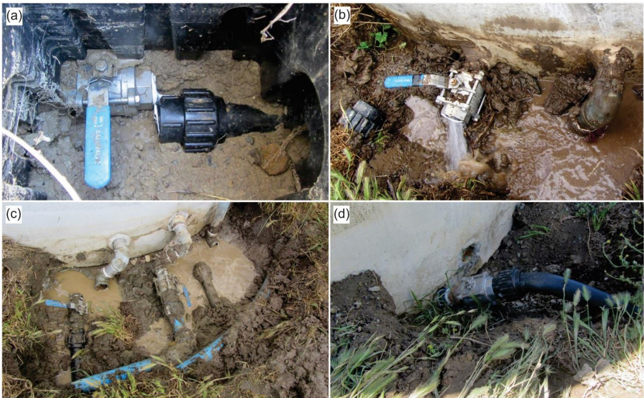
Figure 5. (a) Blind River Tanks. Failure failed threaded fitting due to horizontal displacement. (b) Flaxbourne, failed threaded fitting (Photo: Marlborough District Council). (c) Flaxbourne, failed threaded fitting and rotated galvanized pipe. The pipes rotated due to lateral ground movement. The seal around the pipes into the tanks has been compromised by the movement (Photo: Marlborough District Council). (d) Wheelers Hill. Pipe pulled out of tank wall due to relative displacement (Photo: Marlborough District Council). See Figure 1 for locations.
