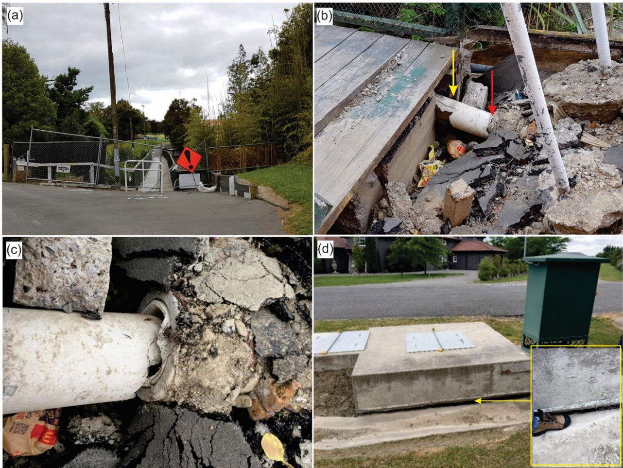
Figure 3. (a) Elizabeth Street Footbridge, Blenheim. The bridge carries a DN100 galvanized steel duct and an Asbestos Cement (AC) water supply pipeline. The galvanized steel duct was deformed and AC pipeline was damaged by displacement of the bridge approach. (b) Elizabeth Street Footbridge. AC water pipe damaged by contacting the concrete pillar (yellow arrow), and has sheared off at the collar (red arrow). Collars under the bridge show evidence of separation. (c), Blenheim. Detail of Elizabeth Street Footbridge AC water pipe sheared off at the collar. (d) Dry Hills Rise, Riverlands. Differential settlement of adjoining components observed in a stormwater pumping station. This is believed to be due to consolidation of poorly compacted fill saturated by rain, rather than by flotation or by liquefaction settlement. See Figure 1 for locations.
