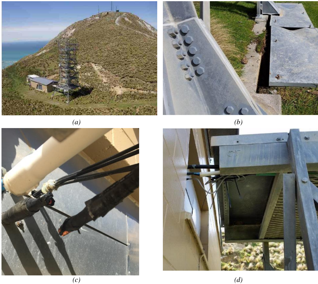
Figure 7: Microwave Station building at Weld Cone, damage: a) building, tower and waveguide bridge between the two; b) permanent ground movement at the tower base; c) broken original coax cable; d) temporary fix for the coax cable (the thin grey cable splicing between the ends of the failed coax cable) and extent of the separation between the building wall and the waveguide bridge caused by earthquake (Photos courtesy of Brent Jones, Chorus).
