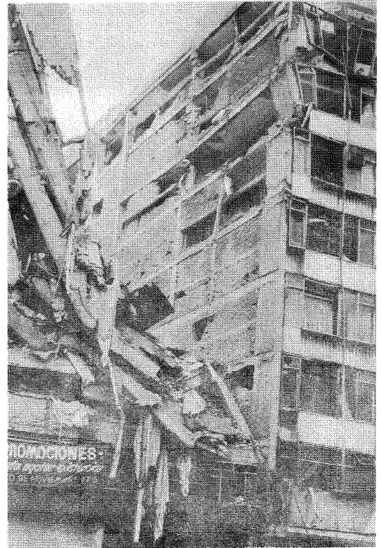
Figure 12 An example of pounding between neighbouring structures with floors at different elevations.
