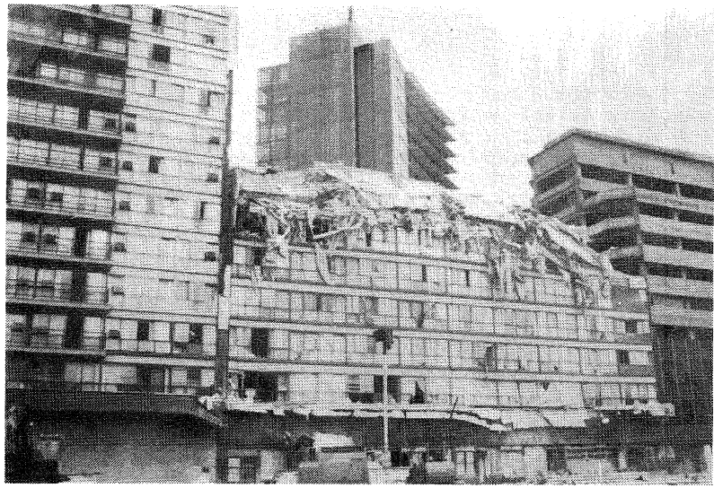
Figure 8 Upper storey collapse in the Continental Hotel.
