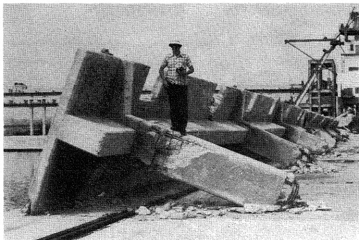
Figure 22 Collapse of conveyor support structure.
