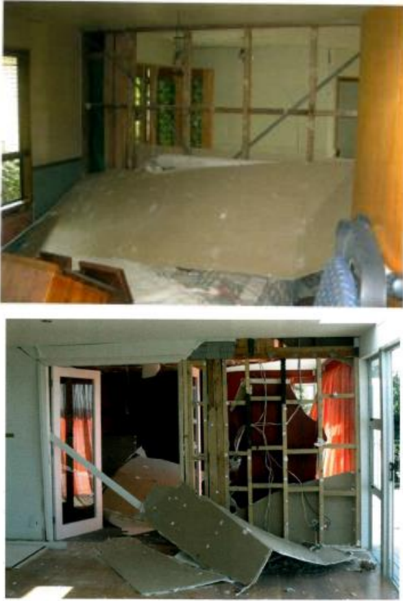
Figure 1: Damage observed in modern LTF buildings following 2010/2011 Canterbury earthquake sequence.
