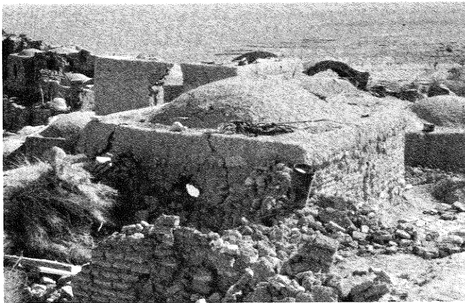
Figure 5. — Damage to adobe buildings.
