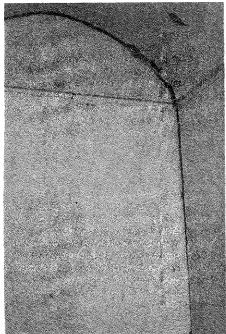
Figure 6. — Damage to newly completed adobe building.
