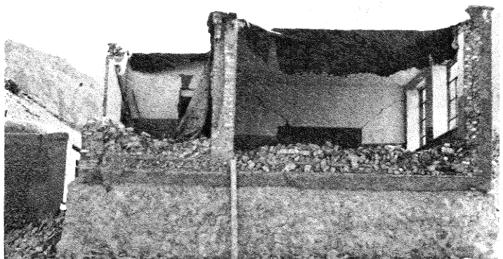
Figure 9. — Damaged brick school.
