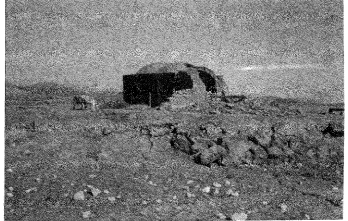
Figure 4. — Damage to domed adobe building.
