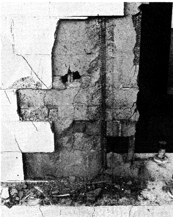
(a) Unconfined Toe, 2 cycles to \mu = 5.5 (Note compression and bond failures)
