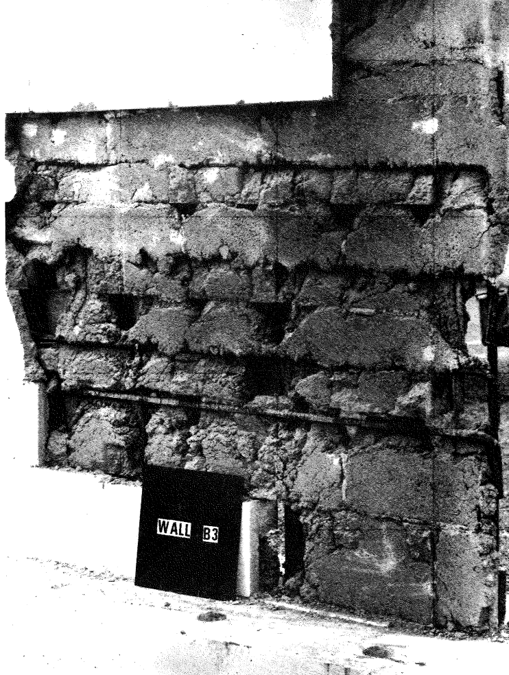
Fig. 2 – Grout core of wall with unsupervised construction, after cyclic in-plane loading.
