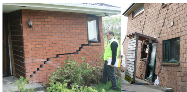
Figure 1: Damage to windows following Canterbury earthquakes.
