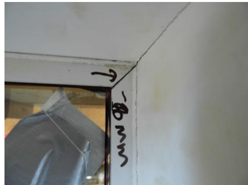
Figure 8: Example of Criteria 1 damage.
