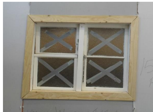
Figure 9: Example of Criteria 3 damage.
