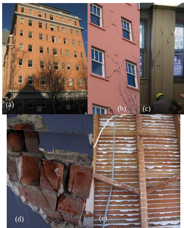
Figure 7: St Elmo Courts seven storeys RC buildings. Shear cracks observed in the masonry infills and column. (Photo Credit: Weng Y. Kam and Stefano Pampanin - (c)).
