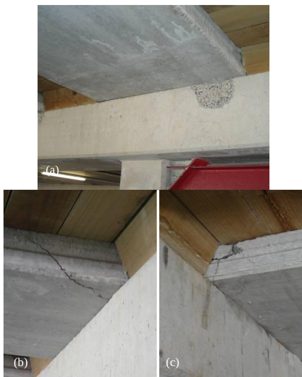
Figure 22: Precast hollowcore floor and seating damages. (Photo credit: Stefano Pampanin).
