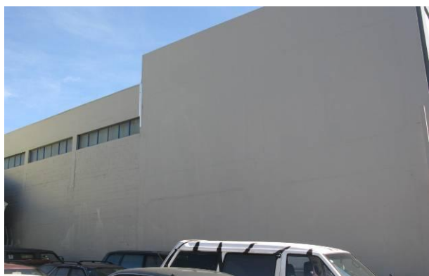
Figure 4: Low-rise pre-1970s RC frames with masonry infills. Separation cracks of the infills and RC frame were observed. (Photo credit: Weng Y. Kam).
