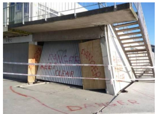
Figure 14: Lateral spreading and liquefaction induced displacement demand resulting in beam-column joint failure. (Photo credit: Charles Roeder).
