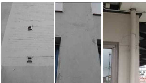
Figure 20: Visible residual cracks in the infills, column and joints (Photo credit: Weng Y. Kam).
