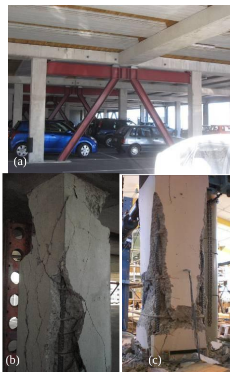
Figure 19: Gravity column failure at car-park structure and similar observation in the laboratory testing by Boys et al. [21]. (Photo credit: top and left: Stefano Pampanin; right: Alistair Boys).
