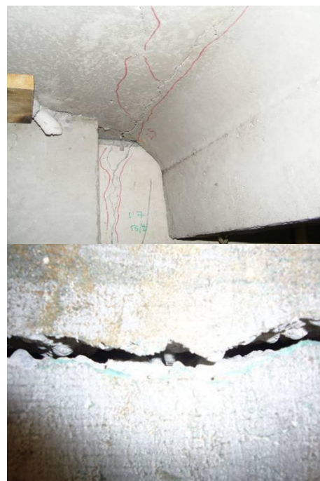
Figure 21: a) Cracks along the T-beam flooring unit perpendicular to the hinging beam; b) Beam-elongation induced slab mesh fracture. (Photo credit: John Hare of Holmes Consulting).
