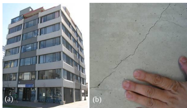
Figure 9: a) Modern mid-rise RC frames building; b) Shear diagonal cracks on modern thick shear walls. (Photo credit: Weng Y. Kam).
