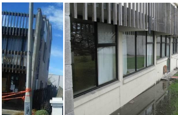
Figure 15: Liquefaction failure-induced tilting and differential settlement of a three storeys RC frames building built in 1978 at Kaiapoi. (Photo credit: left: Rajesh Dhakal, right: Weng Y. Kam).
