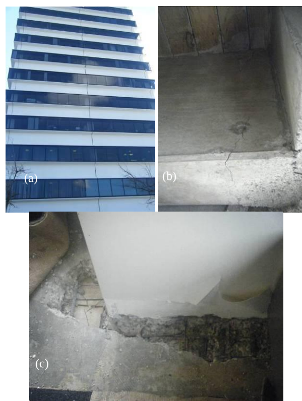
Figure 11: Twelve storey RC frame building beam plastic hinges. (Photo credit: Rajesh Dhakal).
