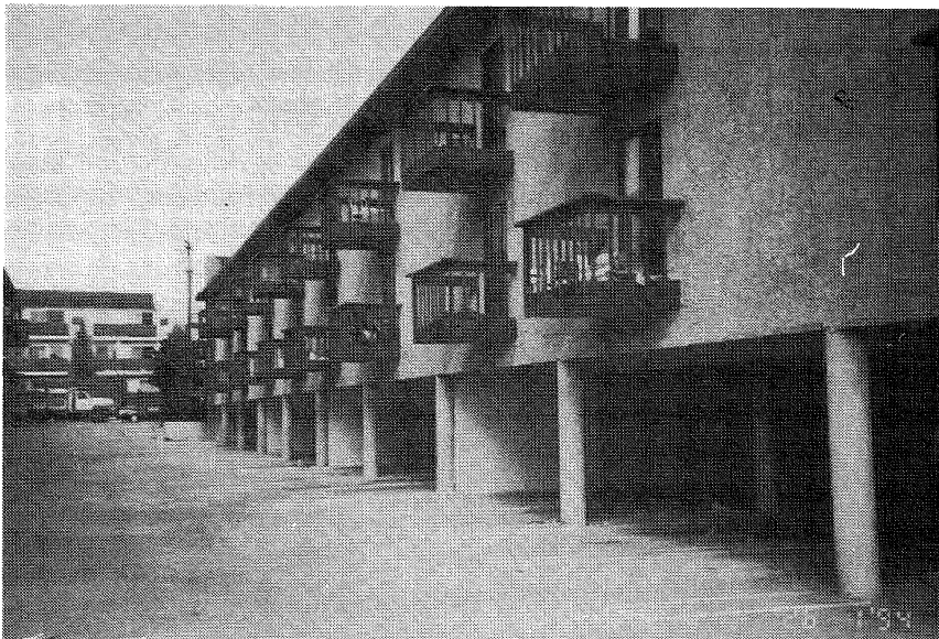
FIGURE 6.50. Concrete support columns damaged but survived (17).
