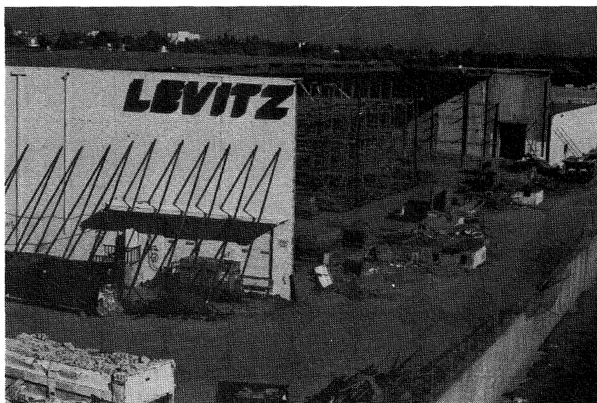
FIGURE 6.25. Levitz Store, Northridge Where both the end roof bay has collapsed and the end wall followed.
