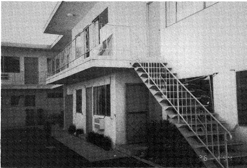
FIGURE 7.6 Olive View Apartments (6). Typical stucco damage to two storey residential units with cracking to lintels and parapets and periodic loss of windows and glass breakage.
