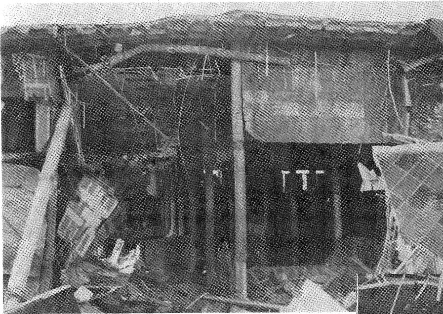
FIGURE 6.2. Bullocks Department Store, Northridge. A forest of columns remains after the punching shear failure of all the floors. Note the waffle slab roof is still in place.
