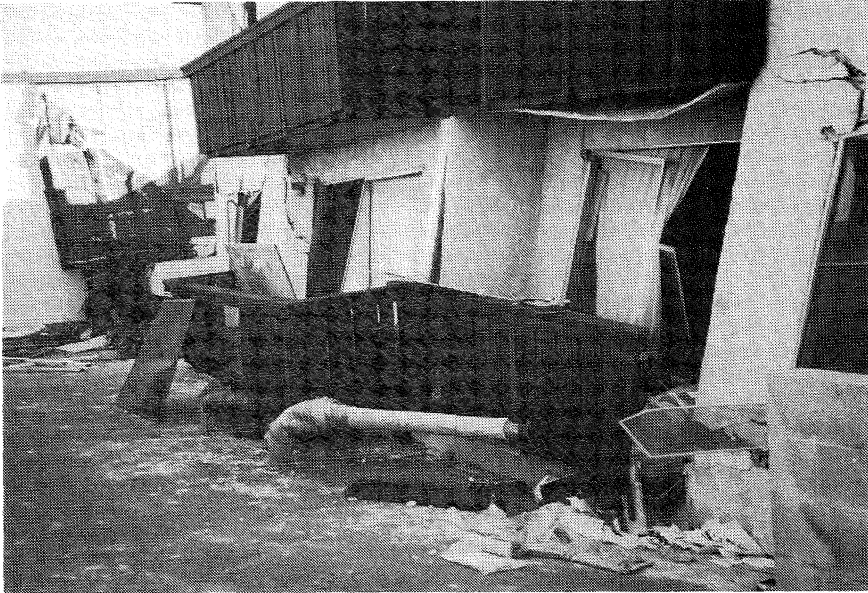
FIGURE 6.54. Meadows Apartments. Rear block collapses with 2.4 m offset
