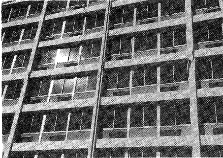
FIGURE 6.6. Holiday Inn, Van Nuys. South side, showing damage zones at Level 4.
