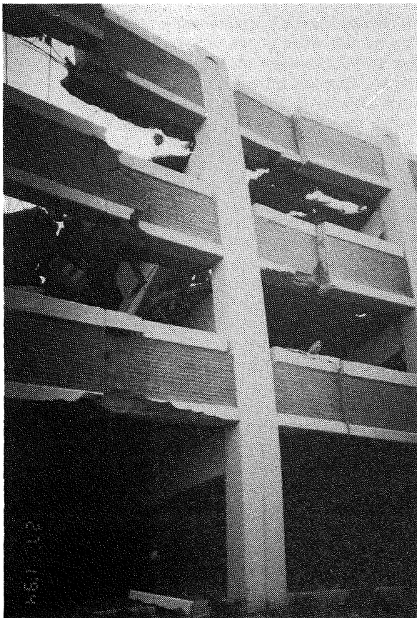
FIGURE 6.32. California State University Car Park. Exterior column/spandrel elements - note mid-span spandrel connection details.
