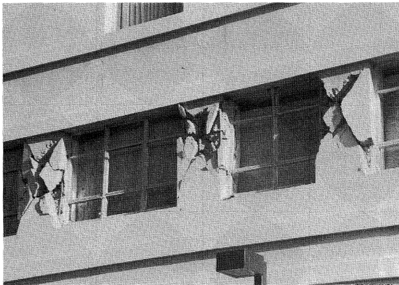
FIGURE 6.14. St Johns Hospital, Santa Monica. Close view of the failed piers (second floor, North Wing).
