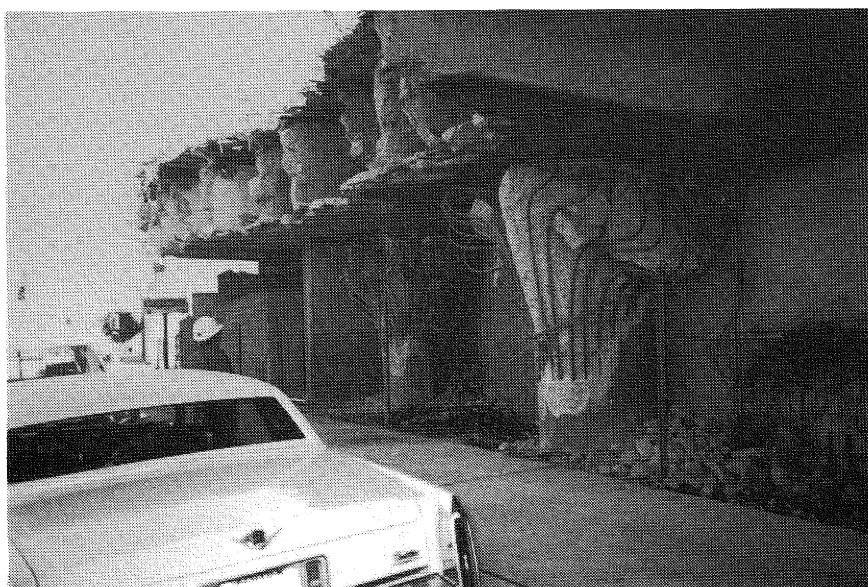
FIGURE 8.19. La Cienega/Venice Boulevards undercrossings of Freeway 10 - damaged columns at La Cienega Boulevard.
