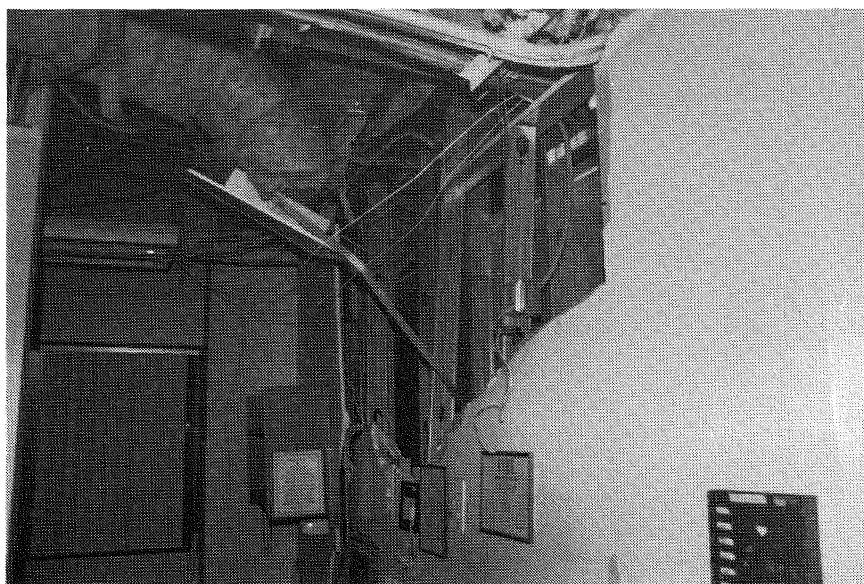
FIGURE 7.11 Holy Cross Hospital (10). Damage to the lift shaft following derailment of the lift car
