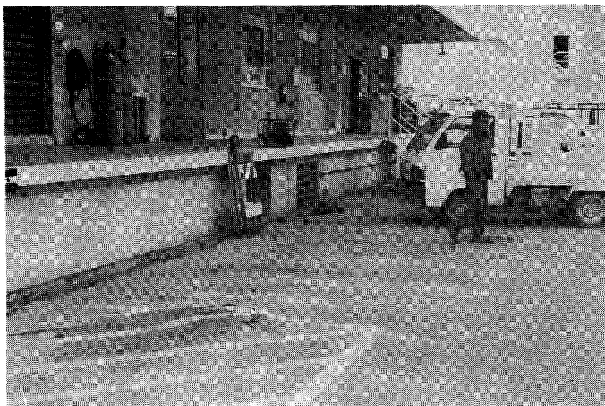
FIGURE 5.5. Settlement adjacent to the control building, Jensen Filtration plant.
