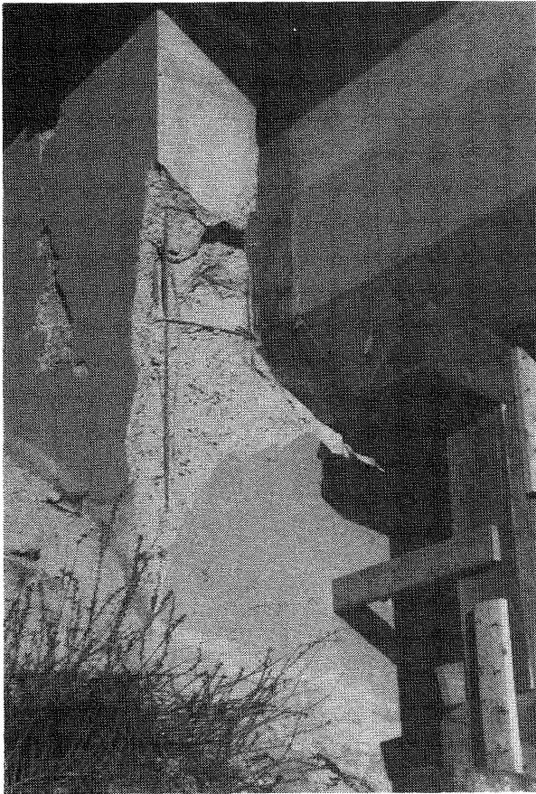
FIGURE 8.8. Interchange of Freeways 5 and 210, eastern abutment showing damaged shear keys and residual box girder displacements of 150 mm horizontal and 100 mm vertical.
