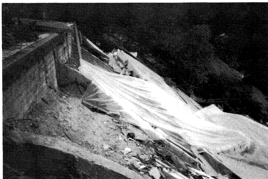
FIGURE 6.47. Sherman Oaks House separated from Ribbon Plate and collapsed down slope.
