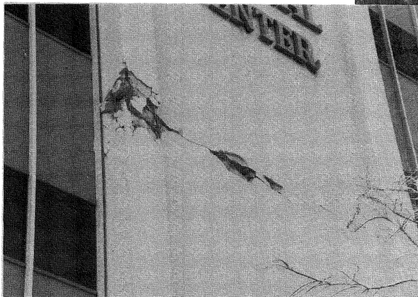
FIGURE 6.17. Indian Hills Medical Center. Failed lap splice in the end zone of the east wall and horizontal construction joint damage.
