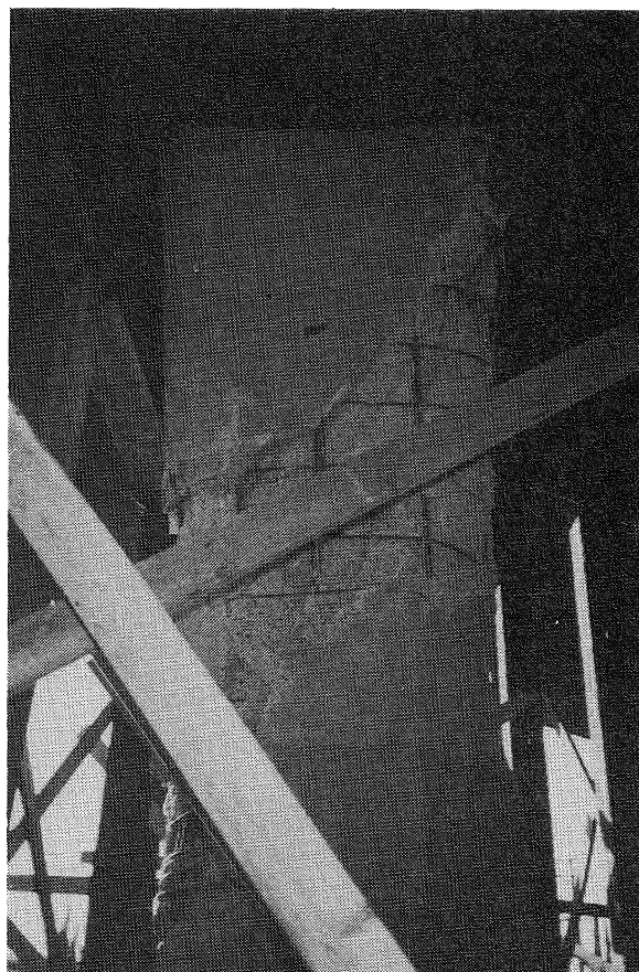
FIGURE 8.13. Mission Boulevard/Gothic Avenue undercrossing of westbound Freeway 118 structure, column 2LR showing concrete spalled over length of column flare, and shear cracking.
