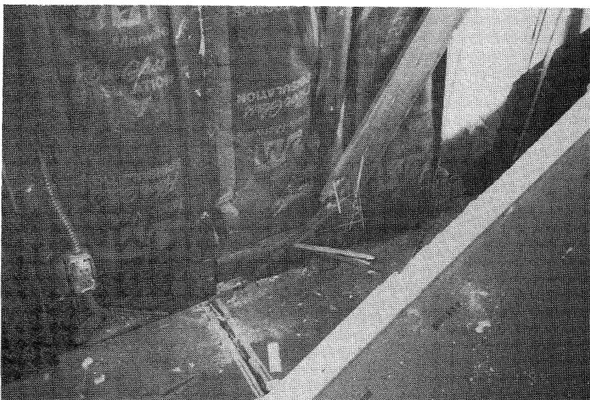
FIGURE 6.56. Meadows Apartments. Cut-in diagonal timber braces failed in compression.
