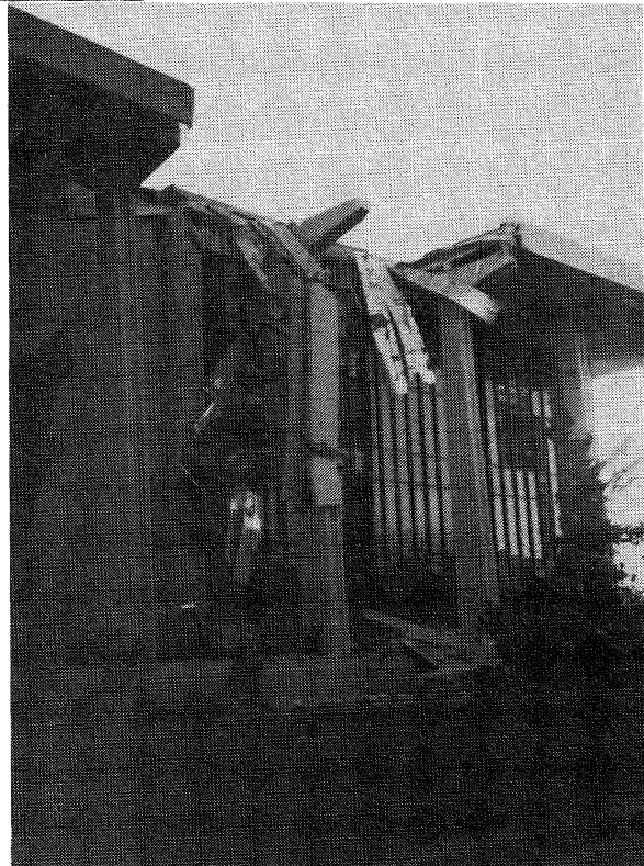
FIGURE 7.3 Oviatt Library (3). Precast concrete parapet panels collapsed consequential to inadequate fixings and high lateral stiffness irregularities.
