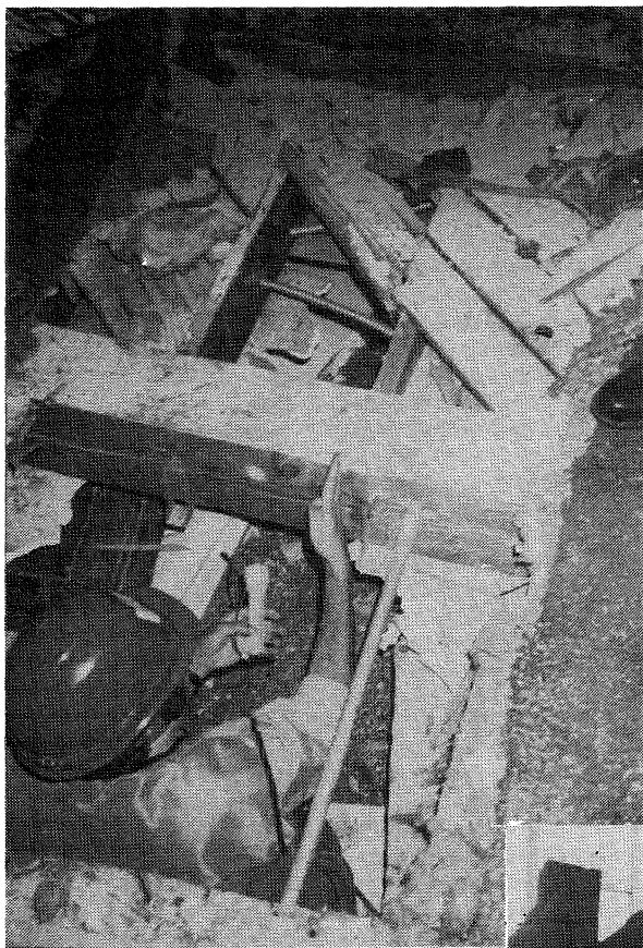
FIGURE 6.57. Meadows Apartments. Evacuation holes cut through the first floor show the floor construction with light-weight concrete topping over diagonal planks with timber joist hanger supports.
