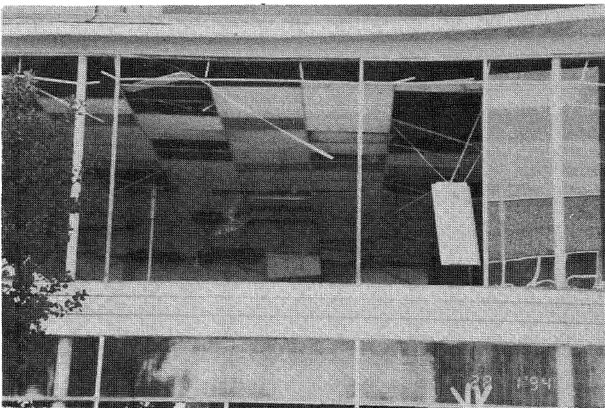
FIGURE 7.12 Retail outlet, Sherman Oaks (11). Suspended ceiling tiles and associated light and air-conditioning vents commonly fell from suspension grids.
