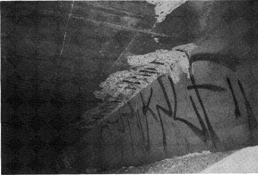
FIGURE 8.10. San Fernando Road undercrossing of Freeway 118, east abutment - spalled concrete at abutment/soffit interface.
