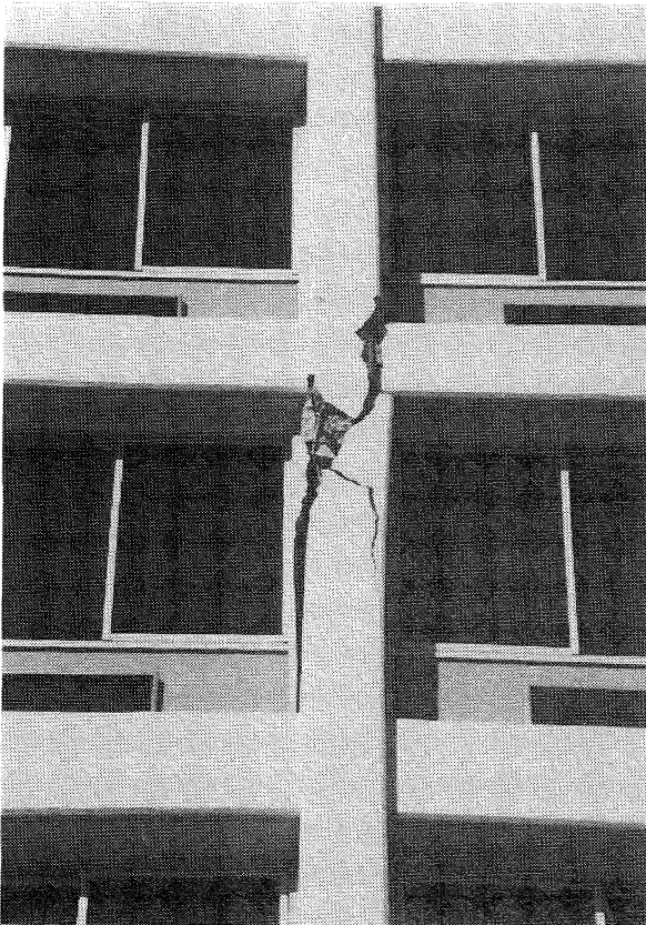
FIGURE 6.7. Holiday Inn, Van Nuys. Close-up of the damage zones at Level 4, south side.
