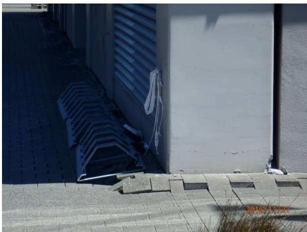
Figure 35: Looking west at southeast corner of the S building at which fill settled approximately 100 to 200 mm relative to pile-supported building. (S41.278285° E174.784757°, 21NOV16).
