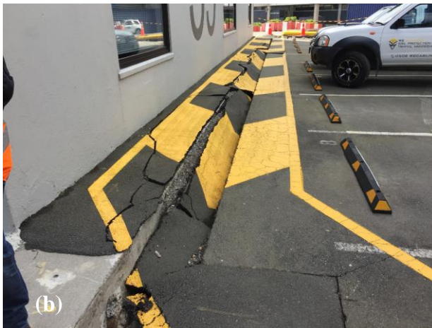
Figure 33: (a) Southeast side of Building S39 and a buried segment of the Fryatt Quay Wharf deck parallel to the building. Fill to the south of the buried mass concrete seawall/wharf settled 220 mm relative to the pile-supported building and wharf deck. ( S41.277984^{\circ} E174.785776^{\circ} , 22NOV16), and (b) looking southeast along southwest wall of Building S39. Fill settled approximately 190 mm relative to pile-supported building at the northwest corner of the building (shown on lower left corner of photo), and magnitude of settlement decreased south-eastward along this wall. ( S41.277994^{\circ} E174.785467^{\circ} , 17NOV16).
