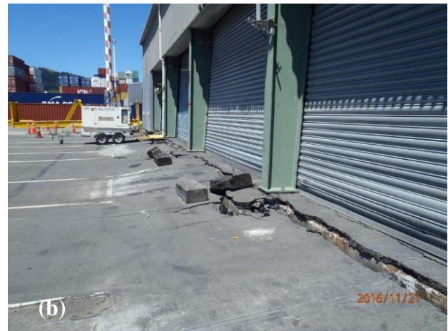
Figure 34: (a) Looking west across north wall of Building S37. Approximately 400mm of differential settlement between ground and deck of buried, pile-supported Pipitea Wharf that supports the western side of the shed. ( S41.278571^{\circ} E174.785632^{\circ} , 21NOV16); and (b) looking south along east wall of Building S37, which shows approximately 375 mm of differential settlement between fill and pile-supported east wall of the building. ( S41.279065^{\circ} E174.785787^{\circ} , 21NOV16).
