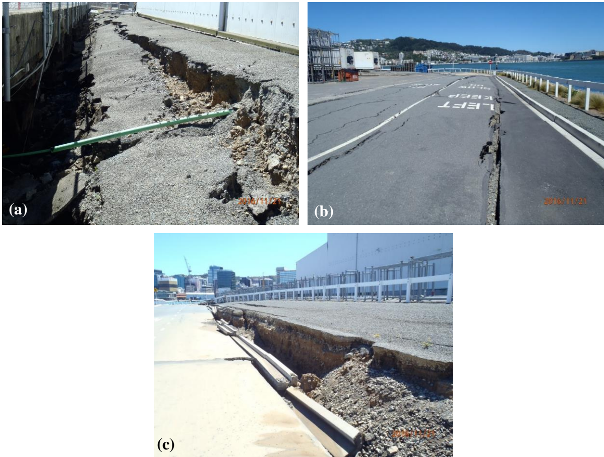
Figure 27: (a) Looking north along the west wall of the CS building. The ground settled approximately 530 mm relative to the pile-supported bulkhead of King's Wharf, which is shown at the left side of the photograph. (S41.280923° E174.784389°, 21NOV16); (b) Ground cracks in area west of the CS building and along the southwestern slopes of CentrePort (looking south). The CS building can be partially seen on the upper left corner of the photograph. (S41.281478° E174.784430°, 21NOV16); and (c) Approximately 1.1 m of vertical offset resulting from the southward lateral movement of the southern edge of CentrePort reclaimed land near its western side. Looking west near the southern wall of the CS building. (S41.281701° E174.785268°, 21NOV16).
