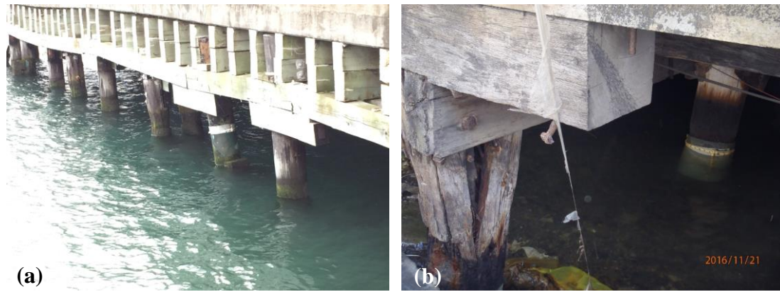
Figure 22: (a) Looking west along southern end of King's Wharf showing westward tilt of piles ( S41.281281^{\circ} W174.784097^{\circ} , taken on 17NOV16), and (b) looking under King's Wharf at an inland bulkhead pile; timber pile is split from lateral movement of the deck relative to the pile. ( S41.280900^{\circ} E174.784375^{\circ} , taken on 21NOV16).
