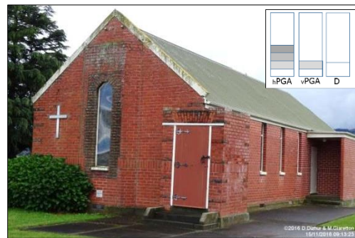
Figure 6: Unreinforced clay brick masonry church in Rapaura, (hPGA 0.269g, vPGA 0.089g – MGCS).
