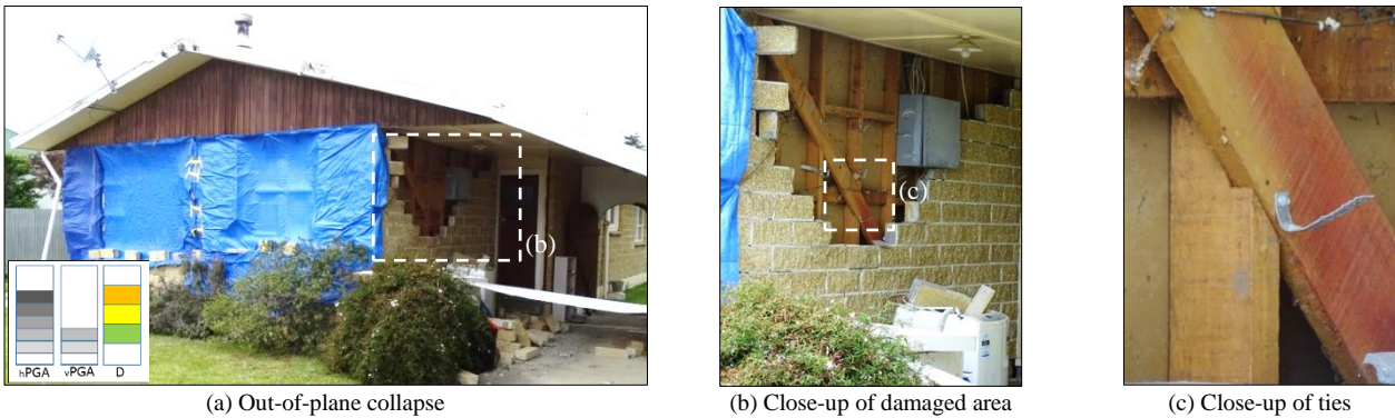
Figure 25: Out-of-plane collapse of masonry veneer in Seddon (hPGA 0.759g, vPGA 0.196g – SEDS).
