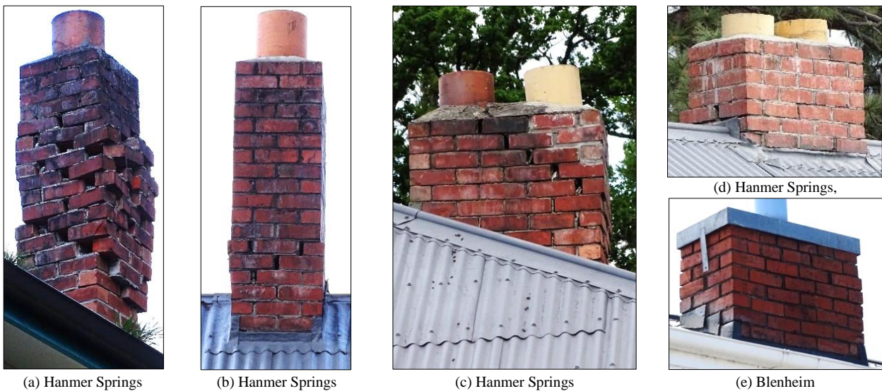
Figure 20: Examples of mortar disintegration and dislodged bricks for chimneys in Hanmer Springs at the historic Queen Mary Hospital and in Blenheim.
