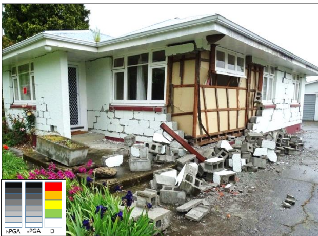
(a) Out-of-plane collapse
