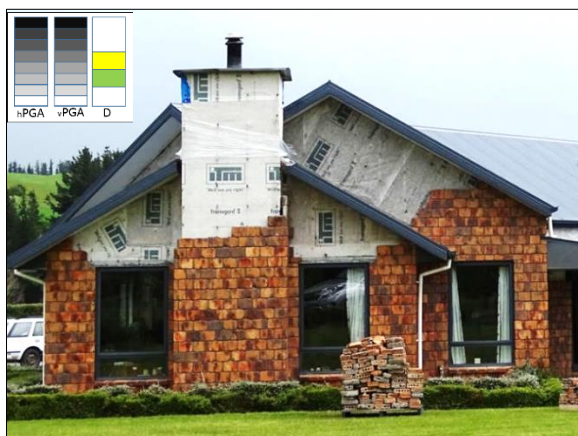
Figure 31: Example of damaged modern masonry veneer dwelling, Waiau ( hPGA 1.124g, vPGA 3.216g – WTMC).
