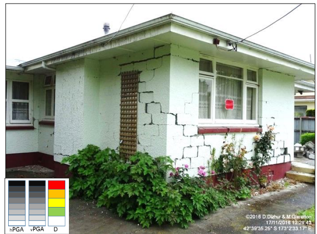
(b) Extensive cracking and dislodged blocks
