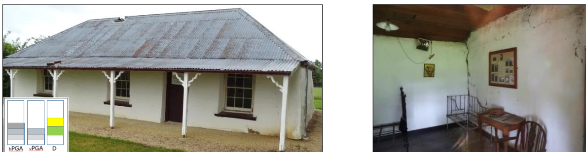
(a) Damage to the Watters Cob Cottage (1885, Heritage List #3691) (b) Internal view showing return wall separation
