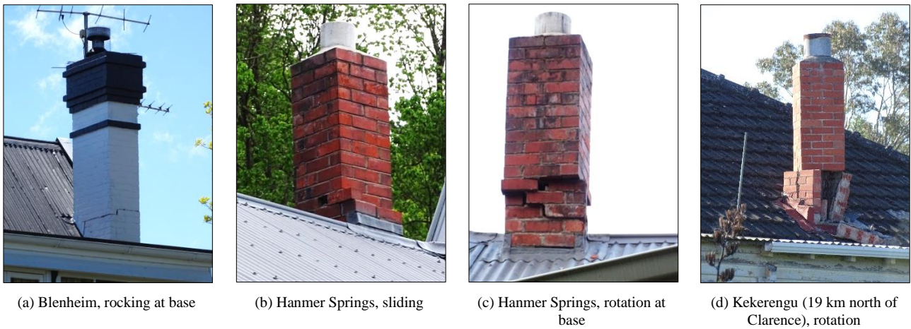
Figure 19: Examples of horizontal cracking at the chimney base with rocking (a) and sliding (b) or rotation (c, d).
