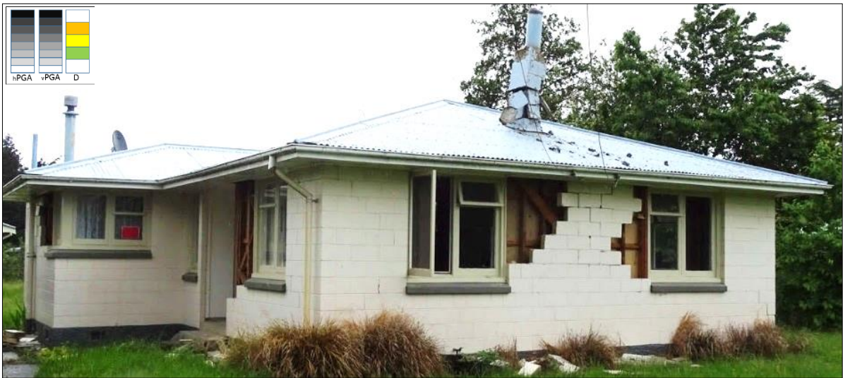
Figure 28: Examples of in-plane and out-of-plane damage to masonry veneer dwelling, Waiiau (hPGA 1.124g, vPGA 3.216g – WTMC).
