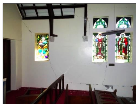
(b) Internal view with diagonal shear and shear sliding cracks
