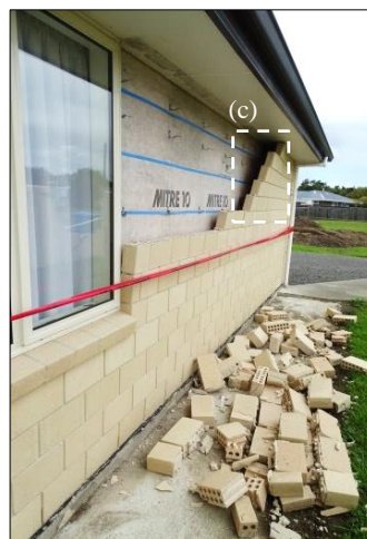
(b) Out-of-plane collapse
