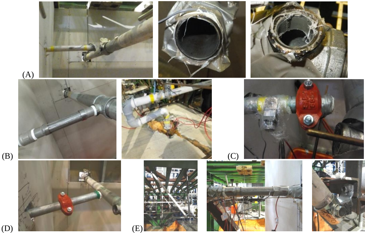
Figure 26: Damage states of each test configuration: (A) OC; (B) FH; (C) CT; (D) CB; and (E) DBF.
