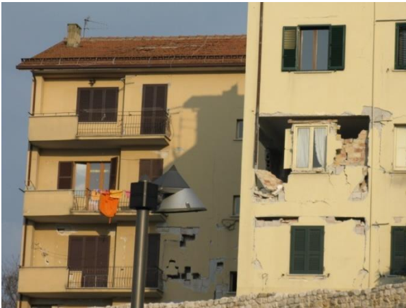
Figure 1: Infill masonry damage observed following the 2009 L'Aquila Earthquake [3].
