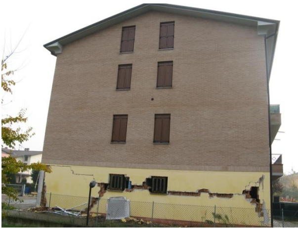
Figure 2: Infill masonry in-plane damage observed following the 2012 Emilia Earthquake [4].
