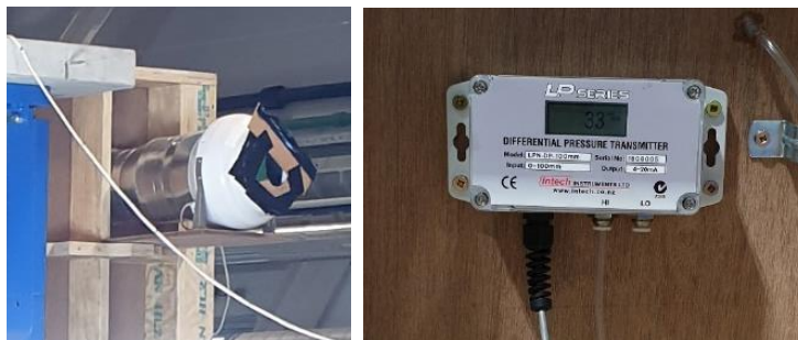
Figure 5: Air pressure control unit. Air blower (left) and differential pressure sensor (right).
