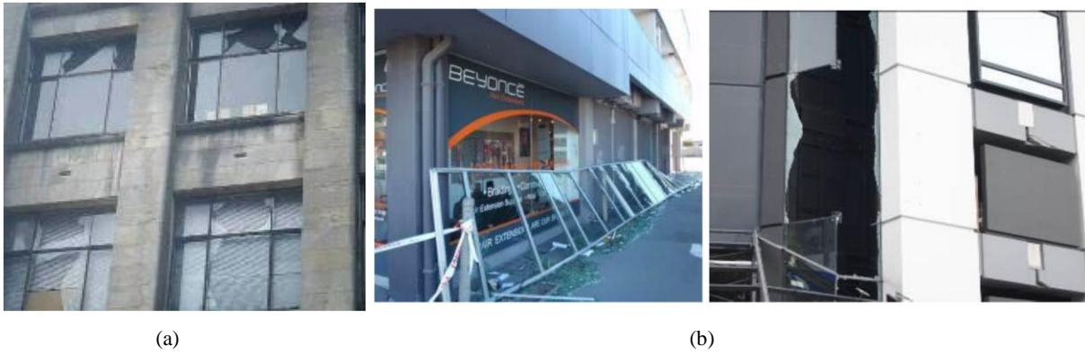
Figure 1: Examples of glazing damage that occurred in (a) the September 4th 2010 Darfield earthquake [1] and (b) the February 22nd 2011 Christchurch earthquake [2].
