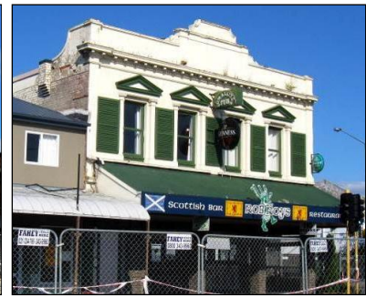
(c) Building B facade condition in October 2010.
