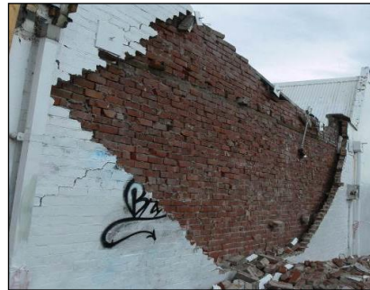
(e) Building C post-22nd February 2011 – collapse of outer leaf of cavity wall.
