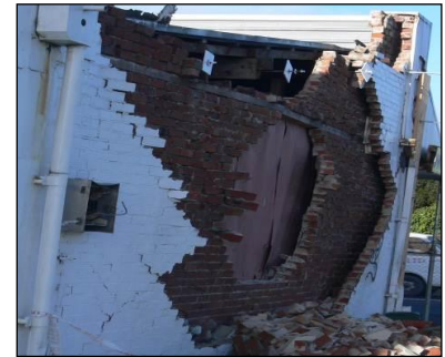
(f) Building C post-13th June 2011 – collapse of inner leaf of cavity wall.
