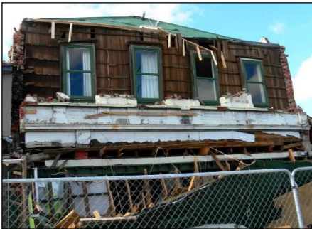
(d) Building B condition in March 2011 – collapse of façade.
