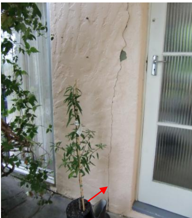
Figure 9: Unreinforced Rammed Earth Kennedy's Bush Road (House 23) showing a minor vertical crack.
