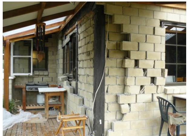
Figure 11: Little River House 17 showing major damage to outer skin of pressed earth brick and significant damage to the inner skin.
