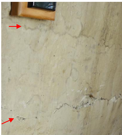
Figure 19: Diamond Harbour house showing the stub wall mid height horizontal cracks due to out-of-plane flexure.
