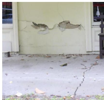
Figure 5: Cracroft House front wall plaster cracks and minor lateral spreading damage to the concrete porch.
