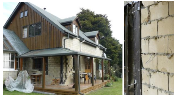
Figure 10: Little River House 17 post and beam construction supporting upper storey, detail view showing ties pulled out of mortar.
