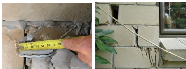
Figure 13: Little River House 17 showing detail of the distorted masonry tie that has failed due to mortar bond. On the right in plane rupture showing mortar failure and crushing of the pressed earth masonry. (G North)
