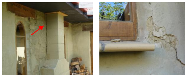
Figure 16: Diamond Harbour reinforced adobe house showing detachment of inadequately reinforced concrete chimney and crack damage at south window.
