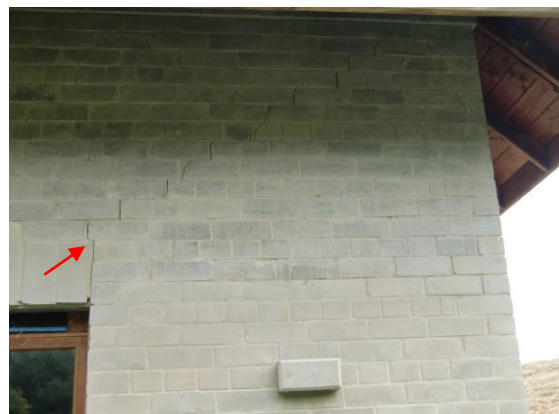
Figure 26: Little River pressed earth house 18 showing cracking of the pressed brick veneer.
