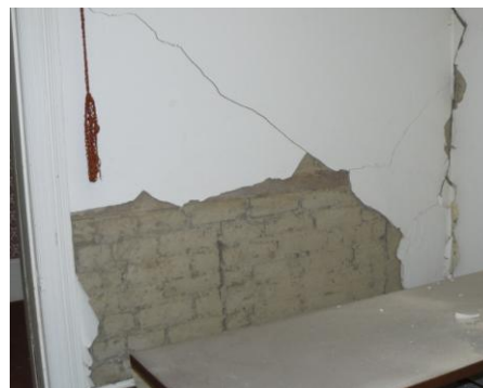
Figure 6: Cracroft House interior plaster with significant damage, underlying adobe wall showing less damage.
