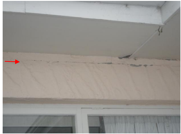
Figure 10: Unreinforced Rammed Earth Kennedy's Bush Road (House 23) showing damage at the bond beam interface over a lintel. (Photo Drupsteen)
