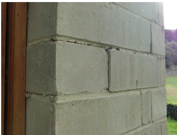
Figure 27: Little River pressed earth house 18 showing cracking of veneer.
