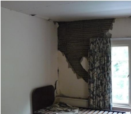
Figure 7: Cracroft House damage to upper level walls of plaster and lath.
