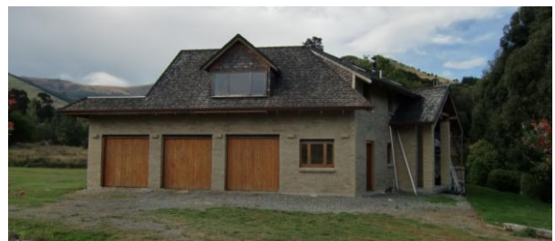
Figure 25: Little River pressed earth house 18 side view showing garages with insufficient adjacent bracing walls. (G North)
