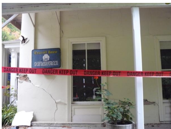
Figure 4: Cracroft House front corner with plaster cracks. The small plaster drop out revealed burnt brick repairs.
