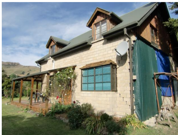
Figure 12: Little River House 17 showing overall house, some minor in-plane cracking and out-of plane failure of the inner and outer skin. (G North)
