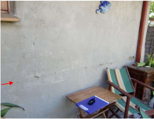
Figure 17: Diamond Harbour house showing cracks on south wall adjacent to entry. (G North)
