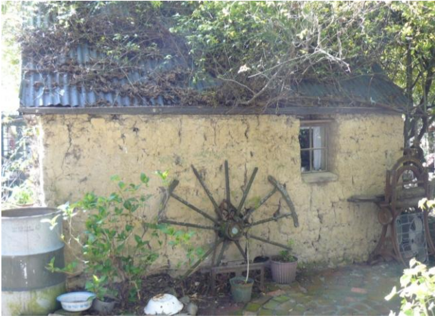
a) Front of cottage showing corner crack at left (surface erosion is also visible).
