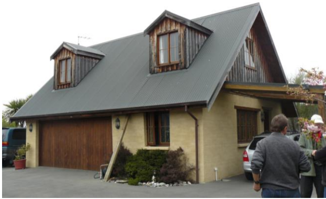
a) Garage with upper level timber, veneer detached adjacent to garage door, significant cracks over end wall lintel.
