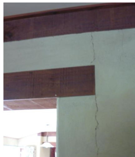
b) Cracks adjacent to the wood faced concrete lintel.
