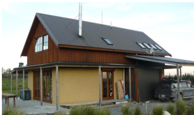
Figure 12: Staveley Adobe House (Building 7) 2008 Structural cracking in short return walls.
