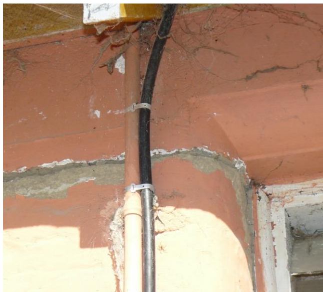
a) Detail of the displacement of the concrete bond beam relative to the unreinforced soil-cement wall.
