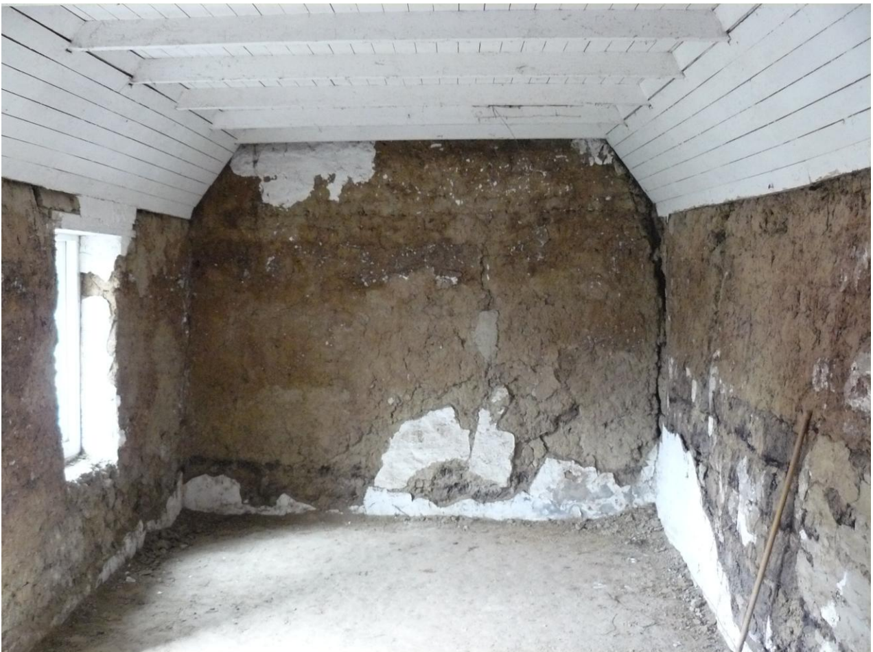
c) Interior showing end wall separation and side wall vertical crack with out-of-plane offset. The interface of the 1860s sod with 1950s cob can be seen on the right hand wall.
