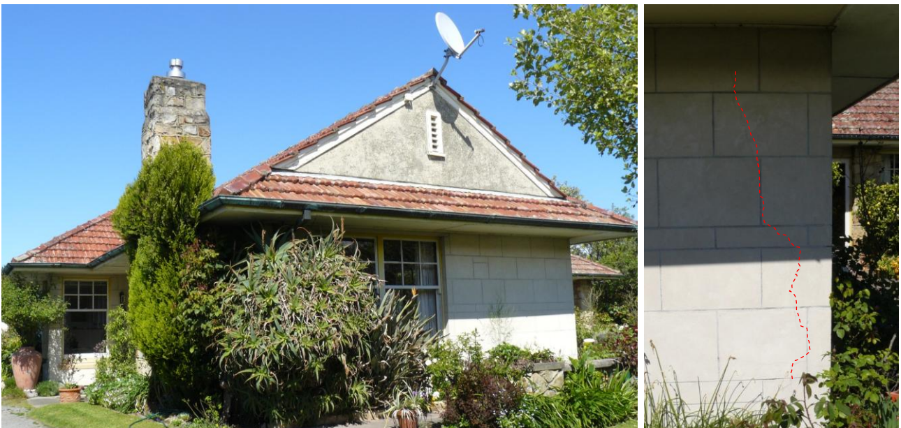
a) Rammed earth house surface plastered – Reinforced concrete bond beam, L shape plan. b) Fine crack full wall thickness.
