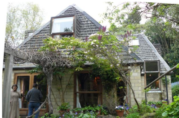
Figure 9: Governors Bay Double Skin Cinva Brick House (Building 8). Subject to strong shaking but with minor damage.
