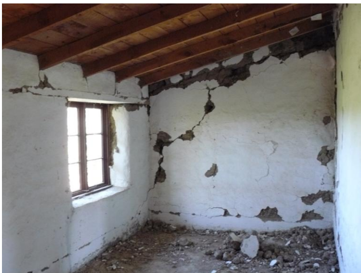
c) Internal view showing complex damage of south wall, east corner .
