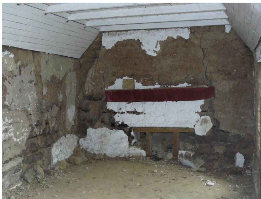
d) Interior damage at the interface with the chimney.
