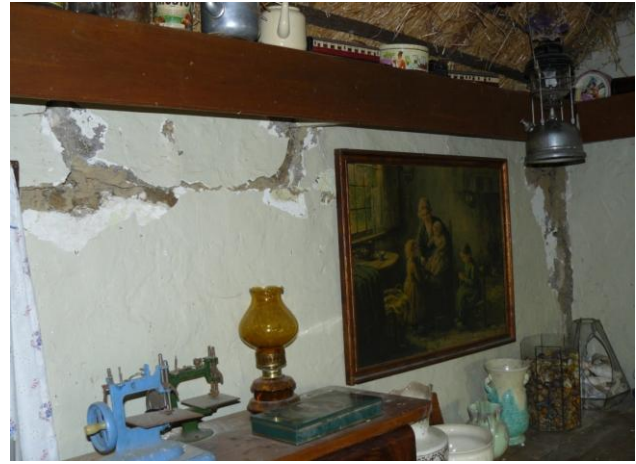
b) Interior of same wall with the corner crack visible.
