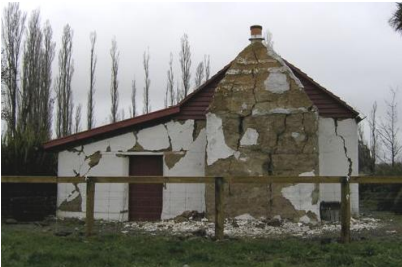
a) North wall of cottage showing major chimney damage after initial event . (Photos John Le Harivel Historic Places Trust)
