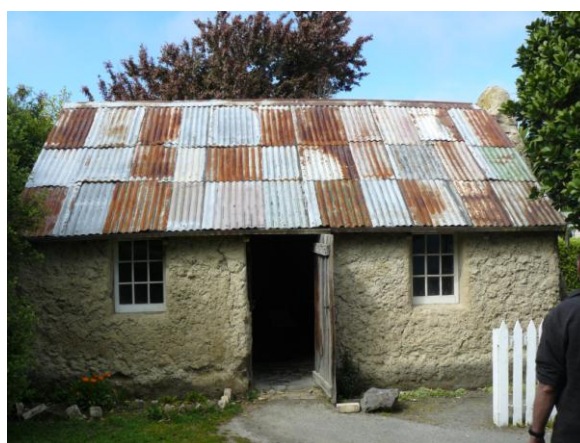
Figure 4: Ferrymead Sod Cottage (building 13) most minor damage was internal – pre-existing crack at doorway opened.
