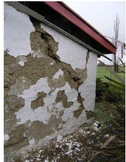
b) South wall, east corner failure.
