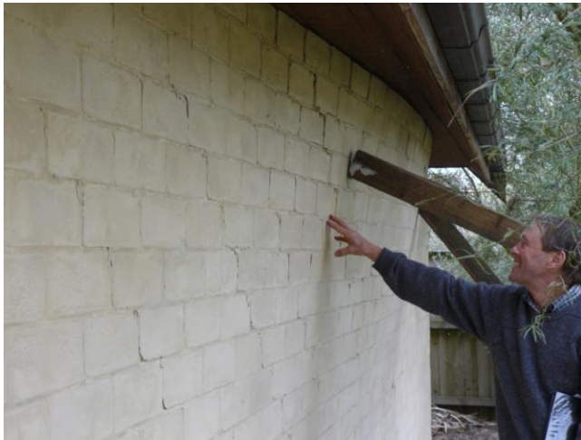
b) Rear wall of garage showing out of plane deformation assumed to be due to veneer ties inadequately anchored into the bricks.
