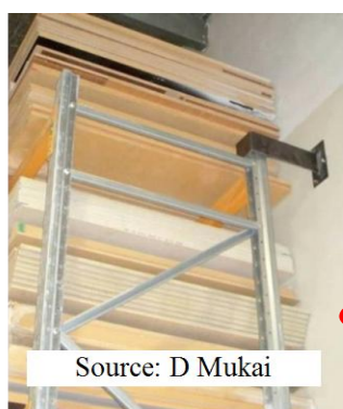
Wall-anchored rack with no damage
