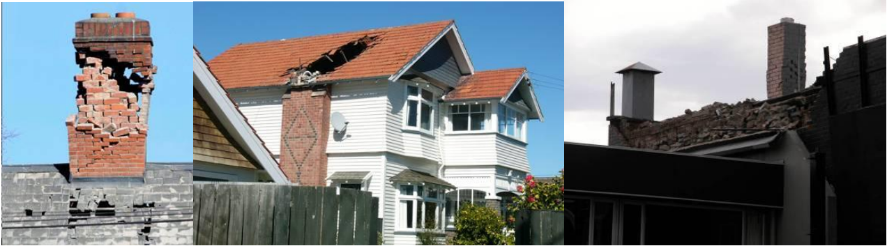
Figure 1: Typical chimney damage.
