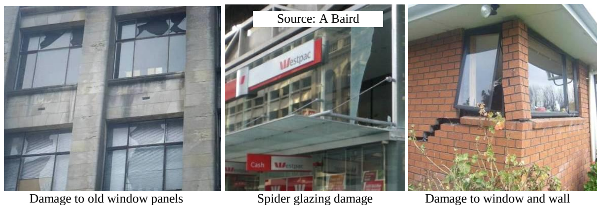
Figure 6: Typical damage to windows.
