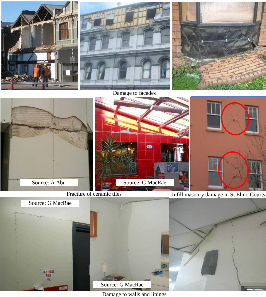
Figure 5: Damage to non structural vertical elements.
