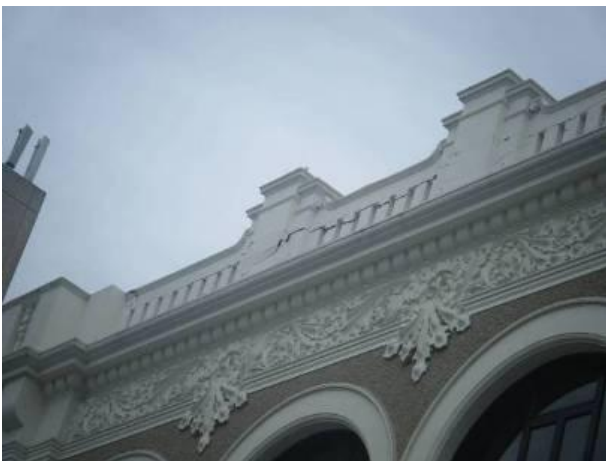
Figure 2: Typical parapet damage.
