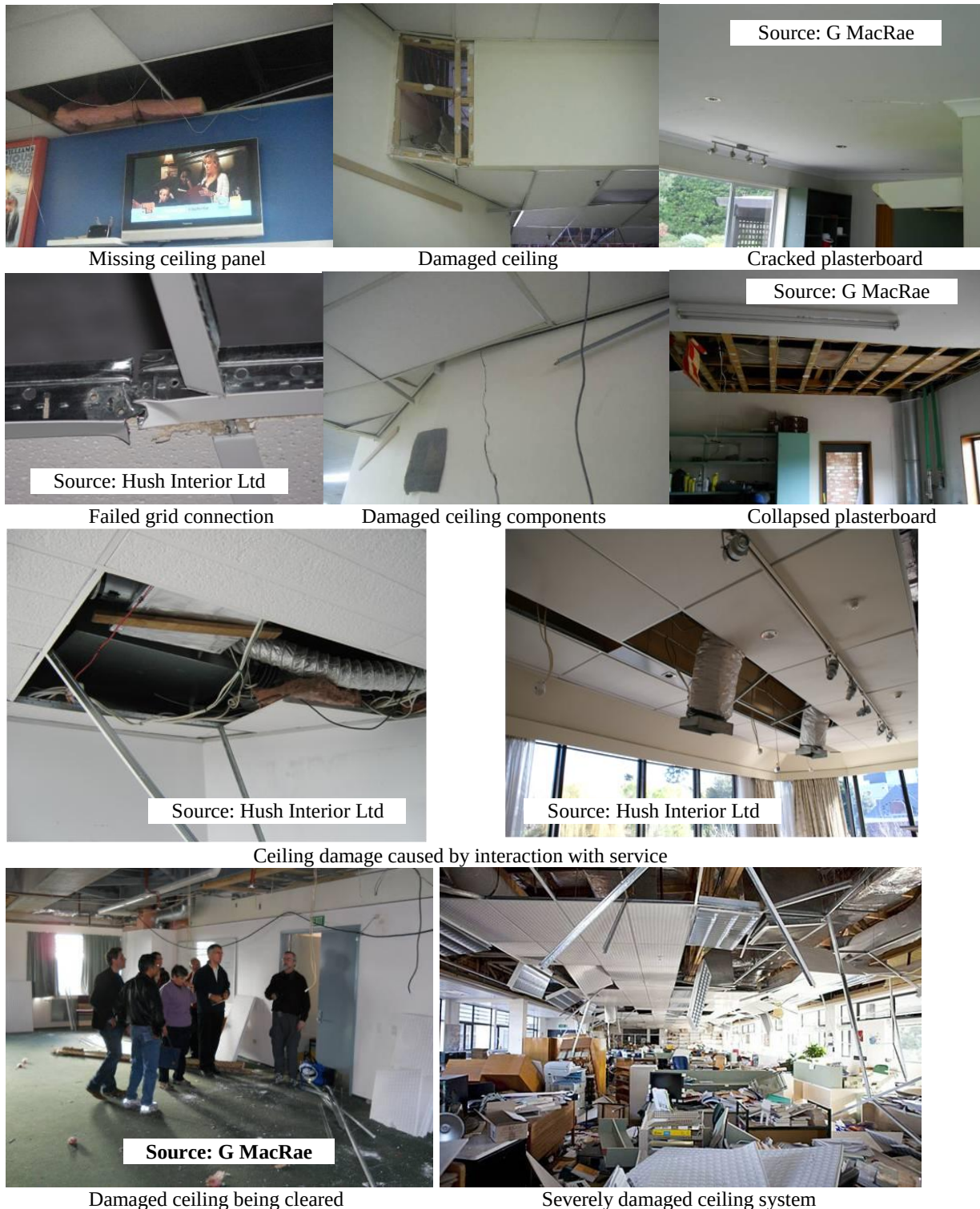
Figure 4: Different types of damage to ceiling systems in residential and commercial buildings.
