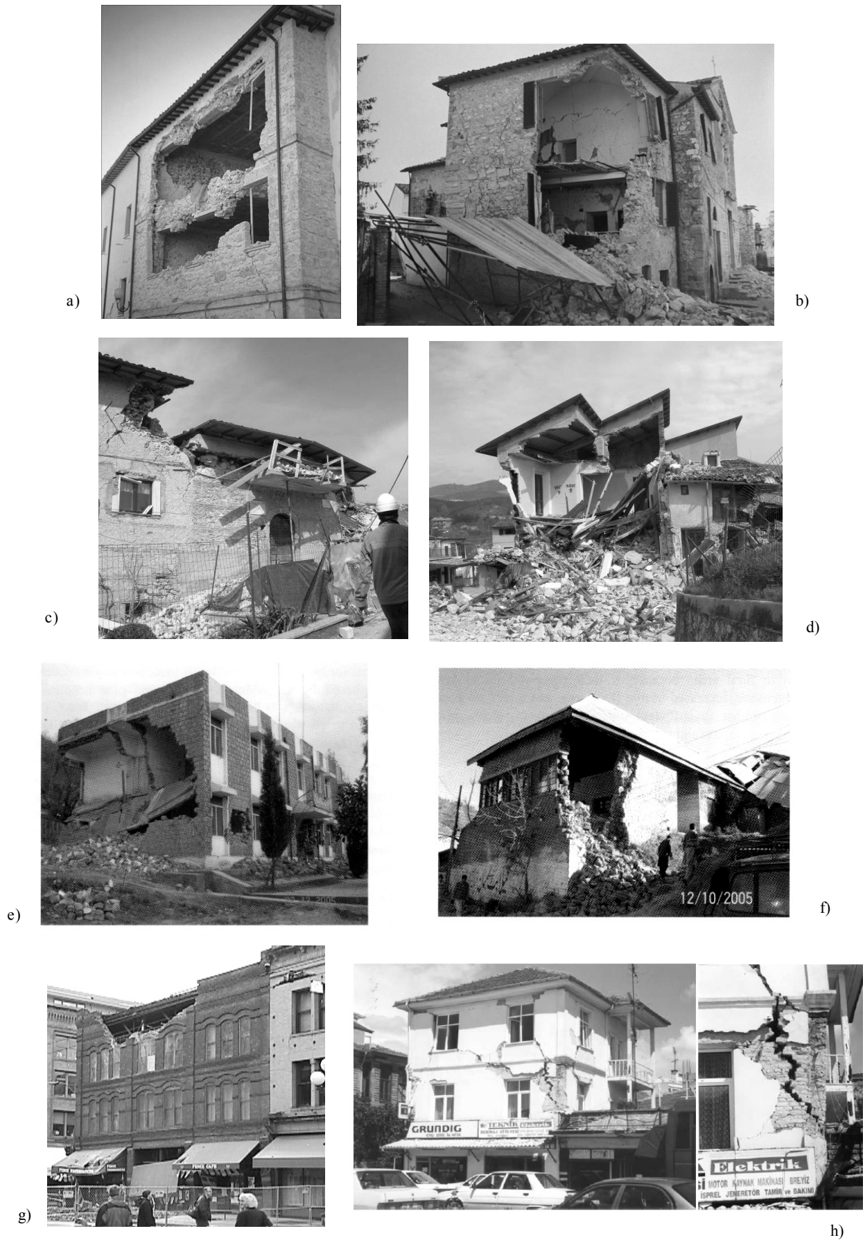
Figure 1: Damages on masonry buildings associated to the presence of inadequately stiff floors observed in different earthquakes in the past: a) 1997 Umbria-Marche earthquake (Italy); b) 2002 Molise earthquake (Italy); c) & d) 2009 Abruzzo earthquake (Italy); e) & f) 2005 Pakistan earthquake (Bothara et al. 2008); h) 1999 Marmara earthquake (Turkey) (Bruneau 2002); g) 2001 Nisqually, WA earthquake (US) ( http://earthquake.usgs.gov ).
